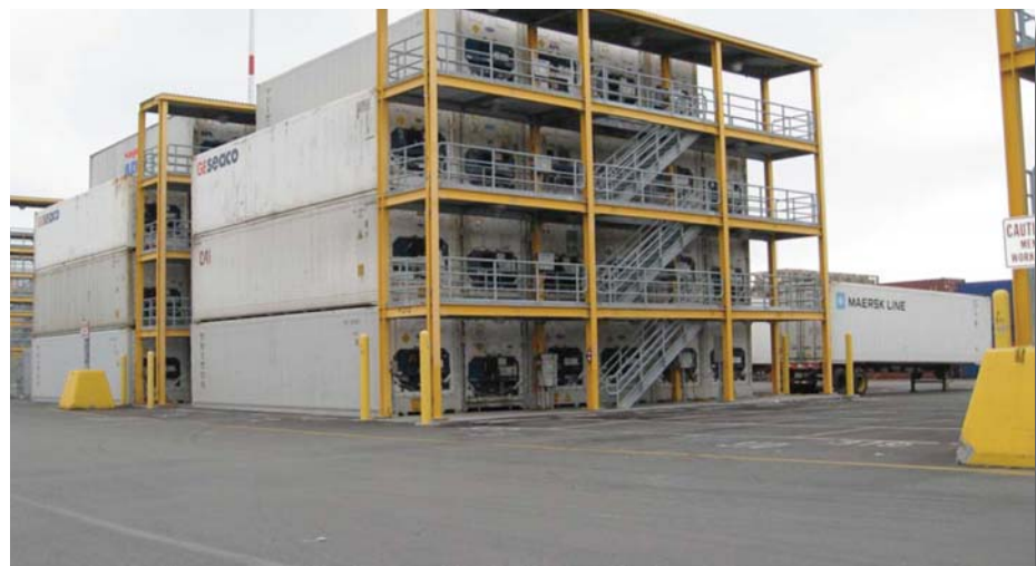
Photo 3: Reefer Rack System (Photo courtesy of John Ryan)
