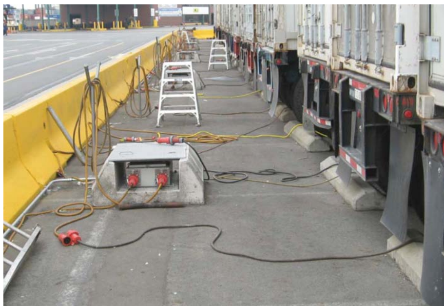
Photo 2: Wheeled Reefers Plugged in (Photo courtesy of John Ryan)
