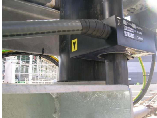
Figure 5-3 HFCT installation to a cable termination
