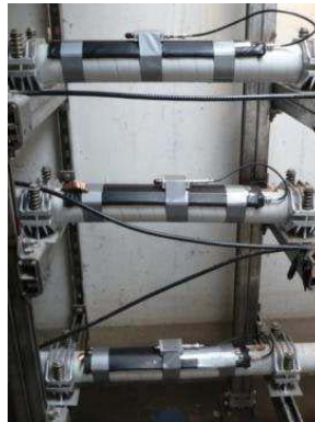
Figure 5-1 Flexible magnetic coupler installed on cable outside jackets
