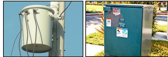
Figure 2 Pole-mounted transformer (left)
