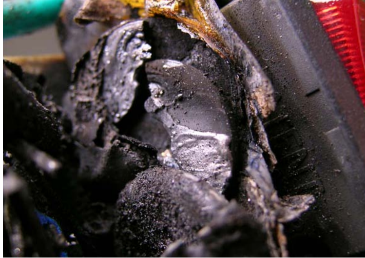
Figure 2-5 MOV Failure Caused by Thermal Runaway and Internal Equipment Fire in another Lighting Controller
