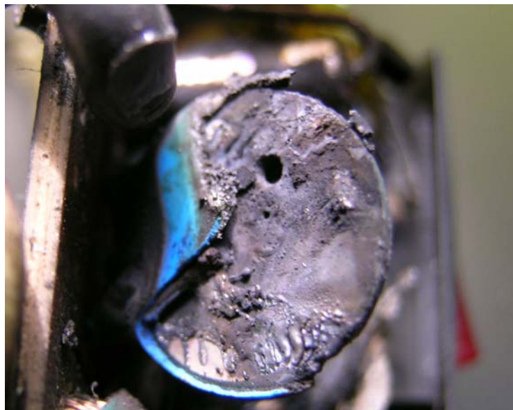
Figure 2-4 MOV Failure Caused by Thermal Runaway and Internal Equipment Fire in a Lighting Controller
