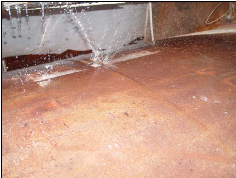
Figure 10-1 Photograph shows the crack in the circumferential weld of the deaerator storage tank
