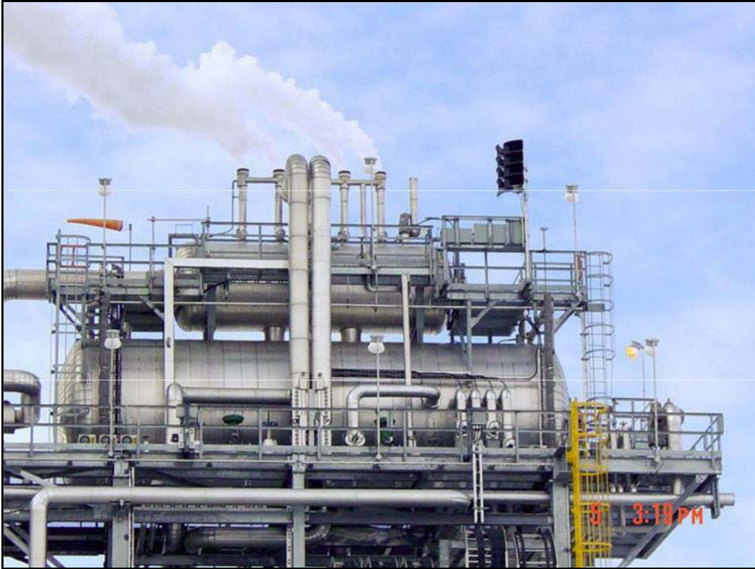
Figure 1-1 Deaerator in operation
