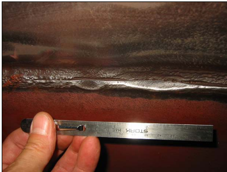
Figure 10-4 Flow accelerated corrosion of the DA heater circumferential weld seam revealed a partial penetration weld. The DA heater was replaced.
