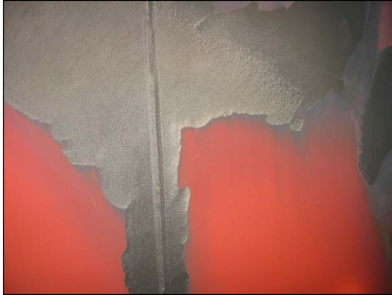
Figure 10-3 Flow accelerated corrosion on the ID of the spray-scrubber deaerator. The circumferential weld was previously ground.
