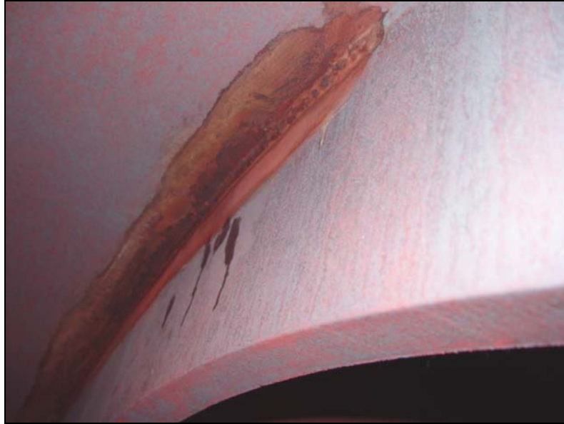
Figure 10-2 Photograph showing the same crack from inside the storage tank
