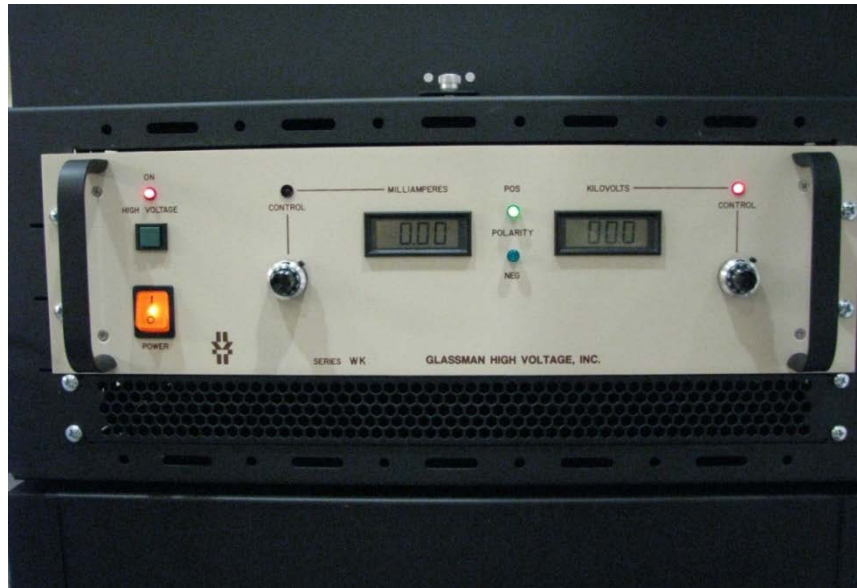
Figure 9-2 DC Test Supply used for Tests
