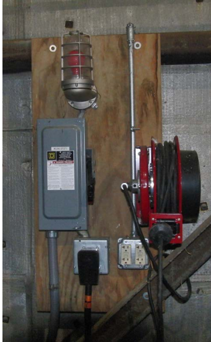
Figure B-12 Breaker on the South Wall of the Building for Energizing the Test Setup with HVAC.
