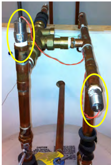
Figure 5-7 Thermistors Installed on Hot and Cold Water Line
