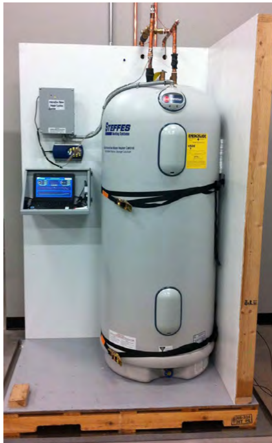
Figure 5-1 Steffes Corporation – Grid Interactive Water Heater
