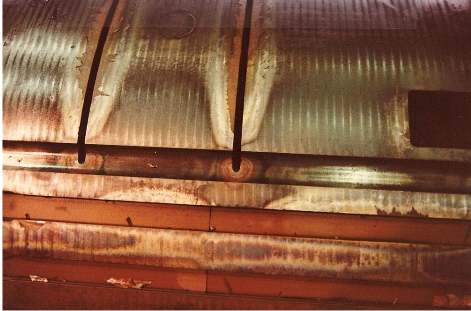
4. Overheating at cross slot
