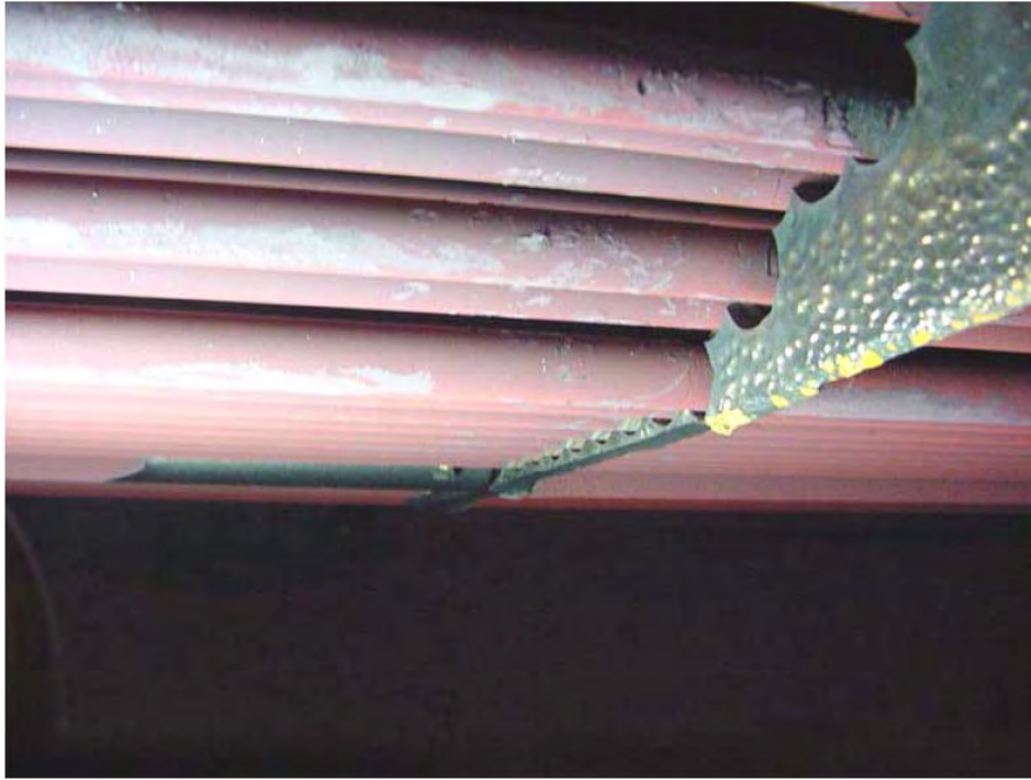
Figure 4-12 Baffle plate degradation
