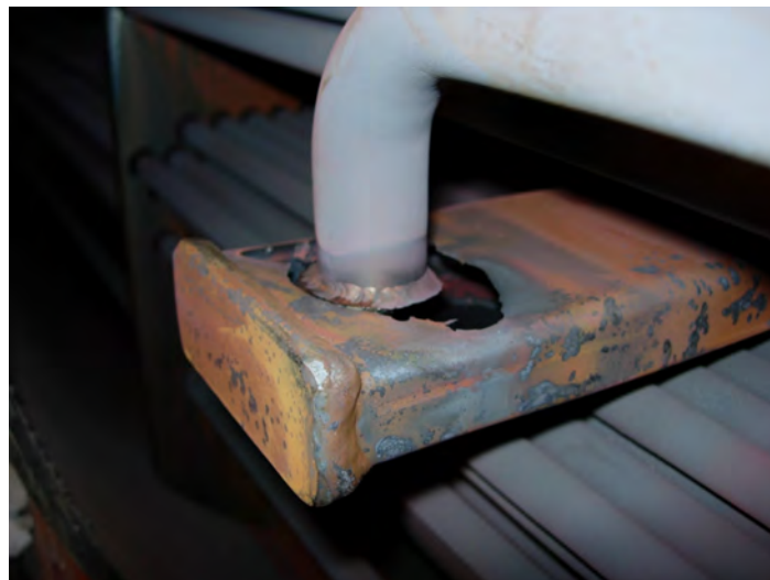
Figure 4-15 Feedwater heater vent manifold failure
