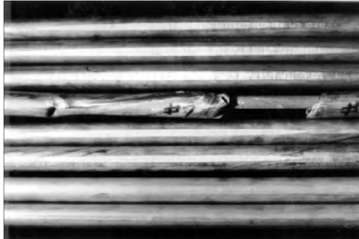
Figure 4-9 Tube-to-tube wear damage adjacent to a tube failure
