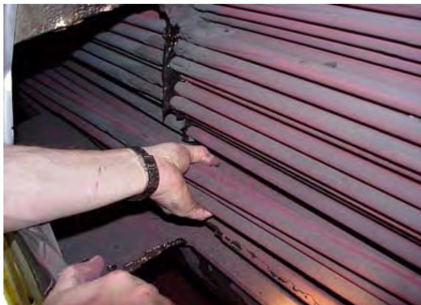
Figure E-2 Missing and partial support plate
