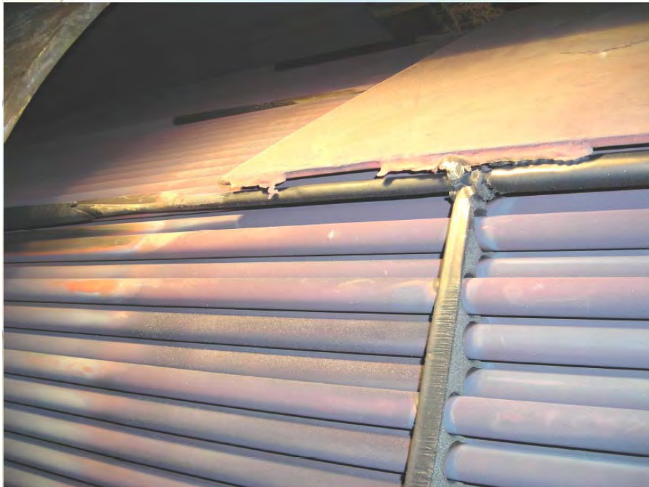
Figure 4-13 Impingement plate with degraded attachment weld
