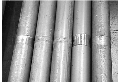
Figure 4-8 Tube wear at support or baffle plates
