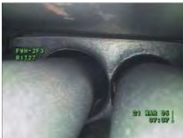
Figure E-1 Example of significant support plate ligament wear
