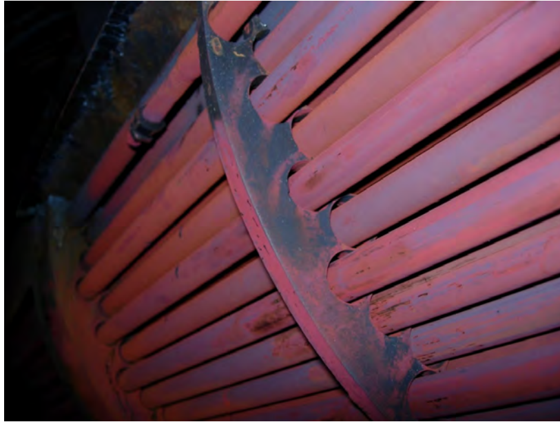
Figure E-3 Partial support or baffle plate due to severe ligament wear
