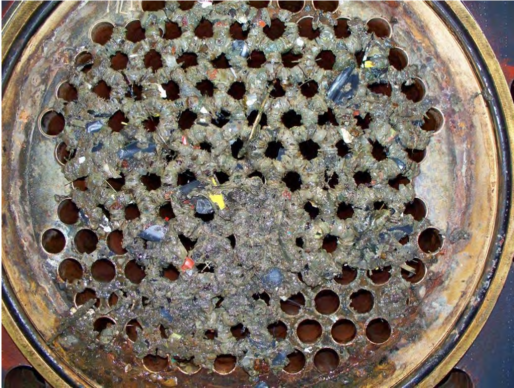
Figure 4-3 Example of macrofouling buildup on tubesheet ligaments
