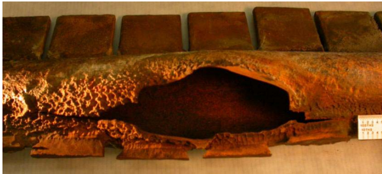
Figure 9-6 Severe corrosion Courtesy of David N. French Metallurgists and Engineers
