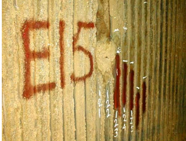
Figure 9-5 Accumulation and erosion to boiler tubing
