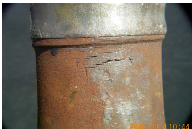
Figure 9-1 A “golden tube.” Finding this problem during an inspection prevents a tube leak that could result in a forced outage.
