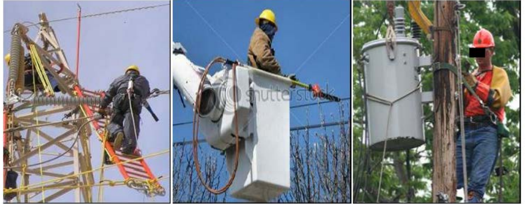
Figure 2-3 Examples of Protective Clothing worn by Electrical Power Workers
