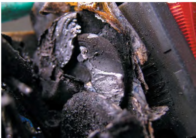
In a surge-protective device, an MOV thermal runaway can lead to a fire inside the protected equipment.
