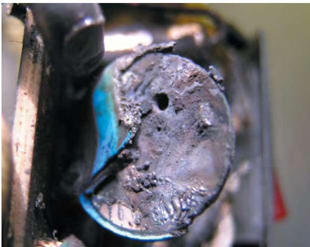
This MOV failure was caused by thermal runaway and fire inside the surge-protective device.
