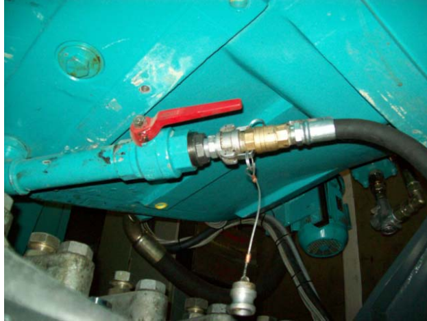
Figure 4-4 Gearbox drain line connection Courtesy of Sage Oil Vac
