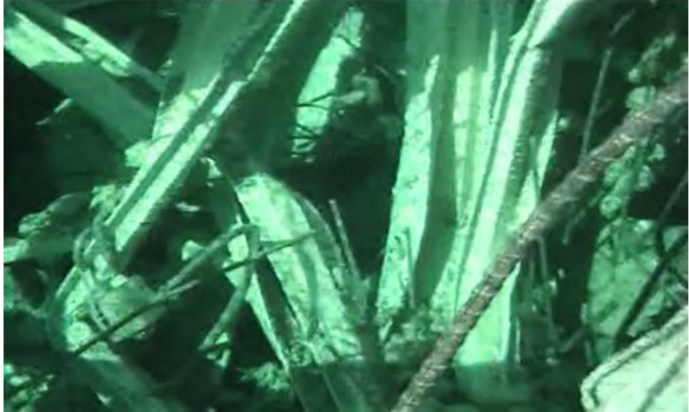
Figure 2-3 Video Image Obtained from Unit 3 Spent Fuel Pool on 8 May 2011. (TEPCO, Copyright 2011. Used with Permission) 33
