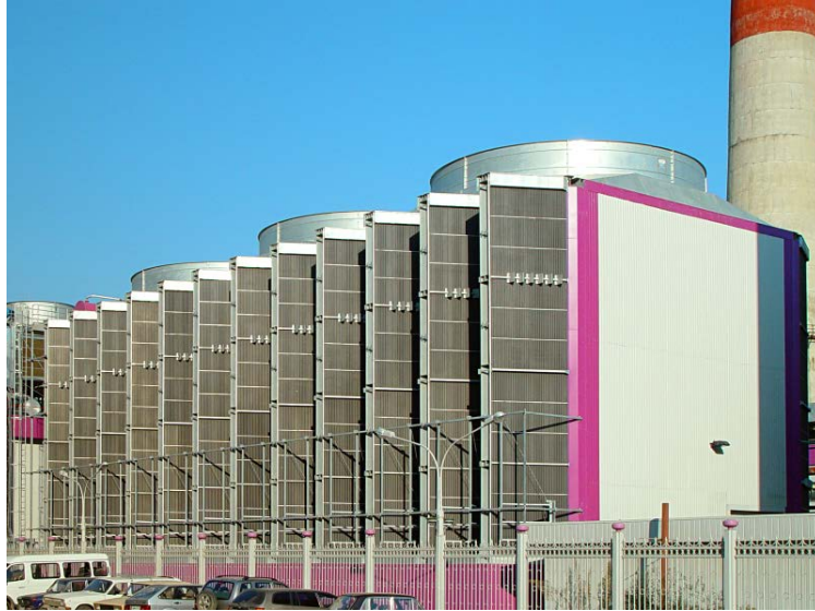
Figure 2-29 Spray enhancement nozzles on mechanical-draft dry tower
