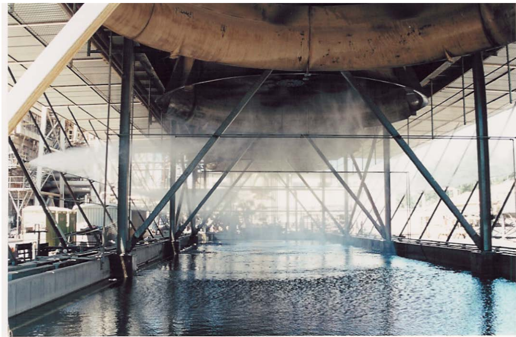
Figure 2-37 Sprays in operation at Chinese Station
