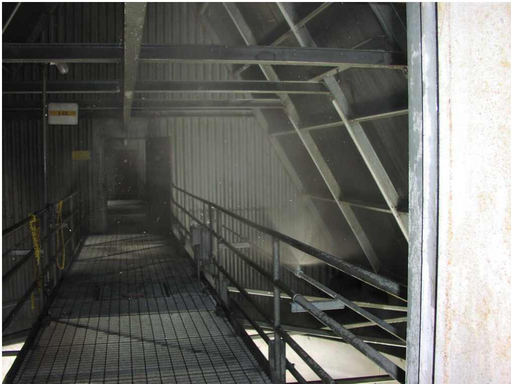
Figure 2-39 Interior spray nozzles in operation at Crockett Co-Generation
