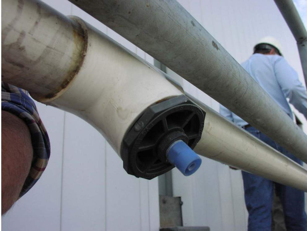
Figure 2-40 Spray nozzle on Linden ACC
