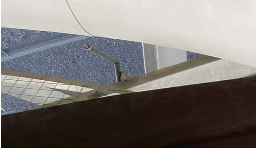
Figure 2-38 Spray nozzle on El Dorado Energy Center ACC
