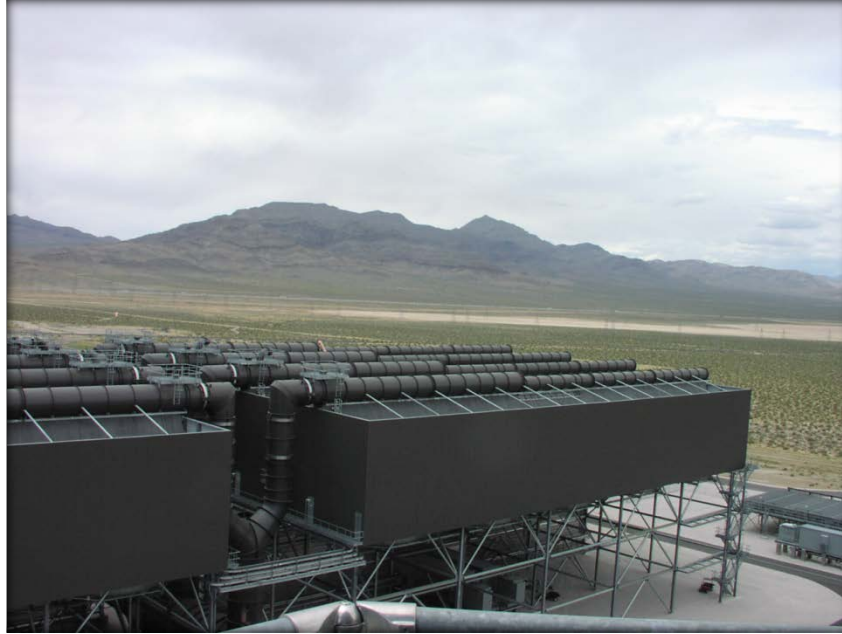
Figure 2-2 View of ACC with Steam Risers, Steam Distribution Manifolds, and Windwall
