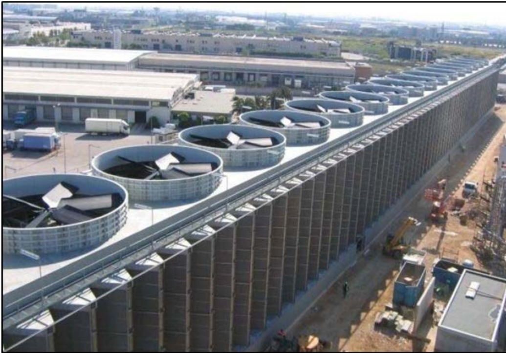
Figure 2-8 Full size ACHE (at Modugno combined-cycle plant, Italy)
