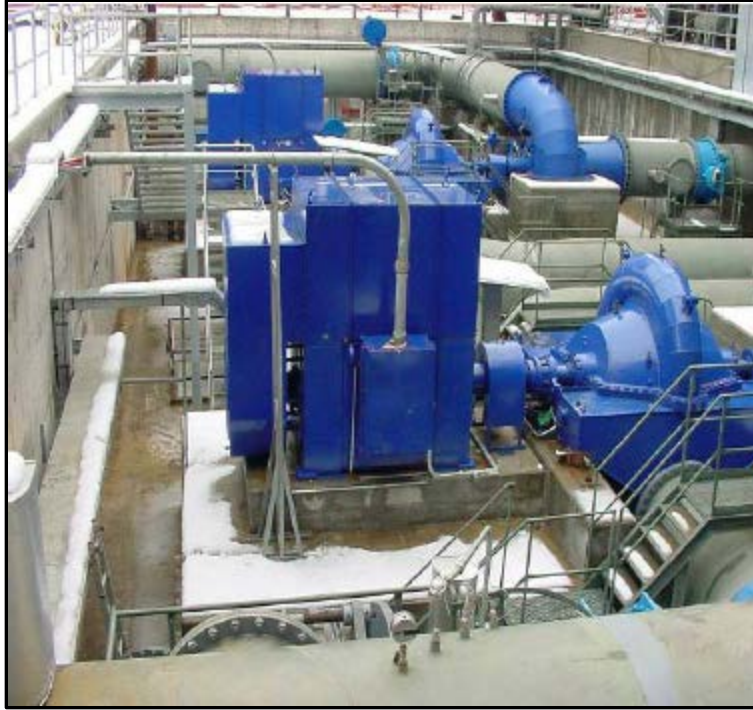
Figure 2-16 Circulating water hydraulic equipment
