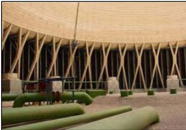
Figure 2-30 Delugeable peak coolers inside natural-draft dry tower
