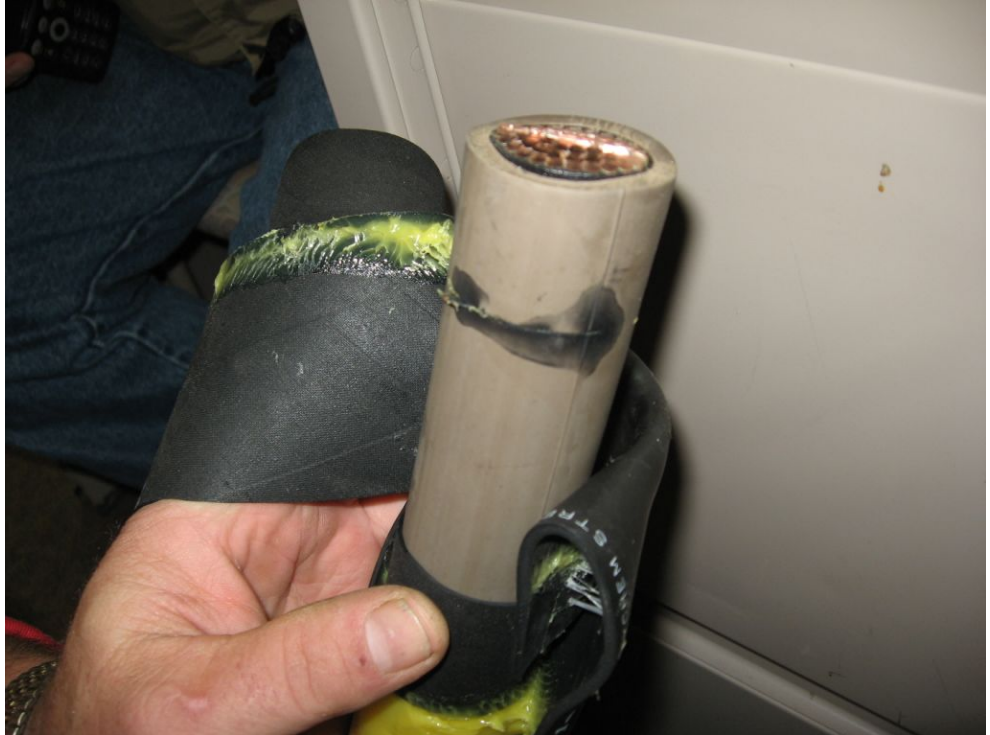
Figure 2-4 Damage to a newly installed cable splice that was identified by a withstand test. The black spot on the cable is where the technician accidentally cut through the insulation when removing the semiconductor shield.
