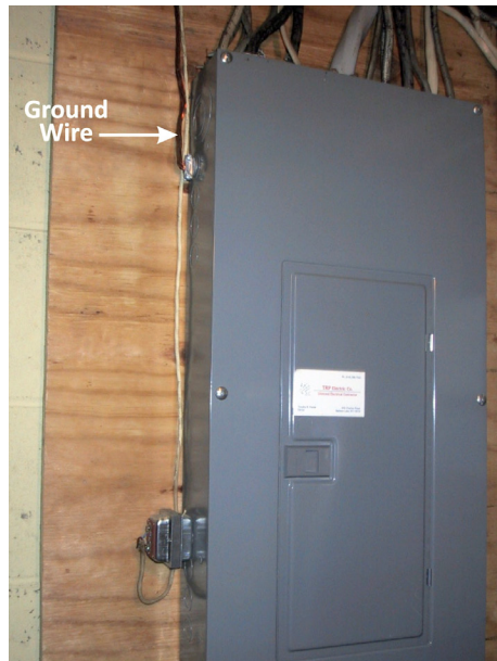
Figure 6. Electrical Panel showing the ground lead at the upper left
