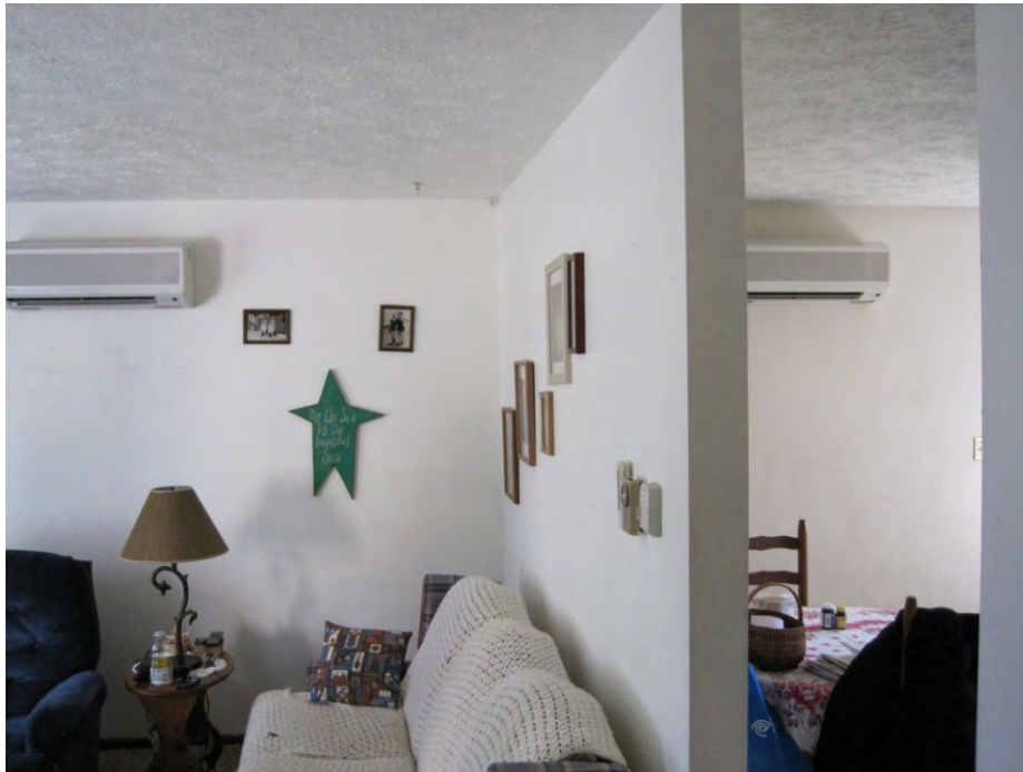
Figure 5-6 Two Zones in a Utility B Site Being Served by Separate Wall-Mount Terminal Units
