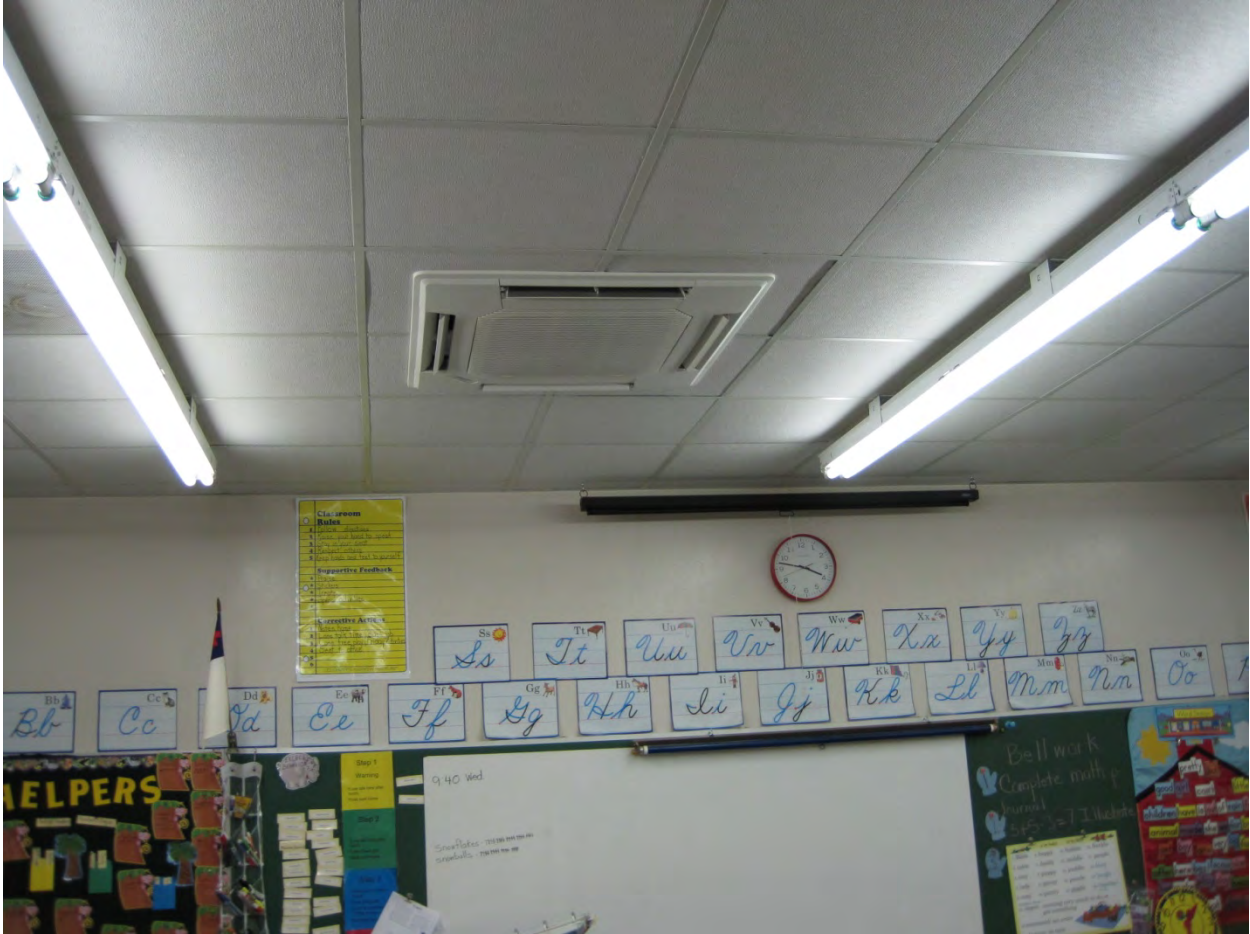
Figure 4-20 Ceiling Cassette-Type Indoor Unit at Site B
