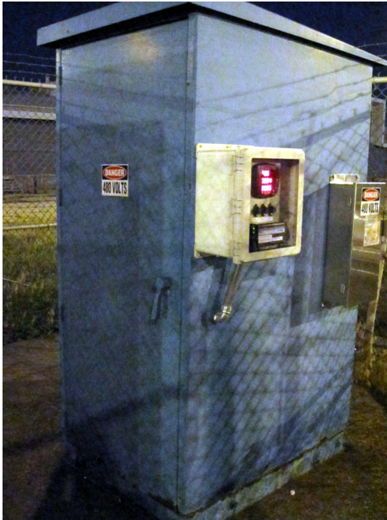
Figure 6-3 An Energy Monitor Installed in a UL 508A Enclosure
