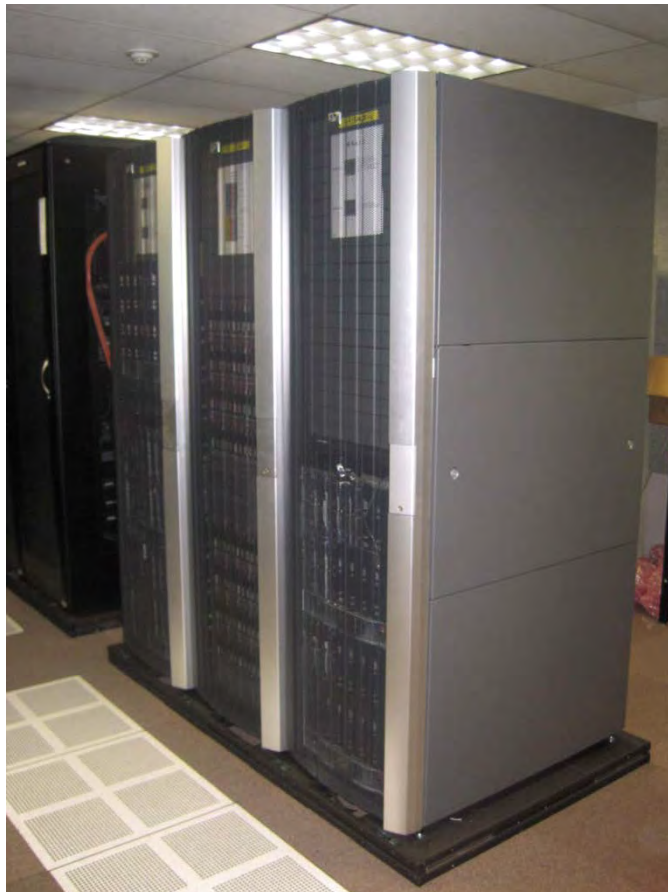
Figure 3-4 A Rack of Blade Enclosures
