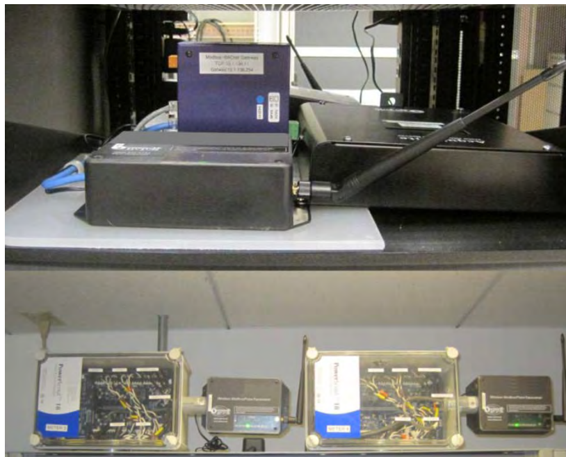
Figure 3-11 Equipment Used to Monitor 22 Three-Phase Circuits
