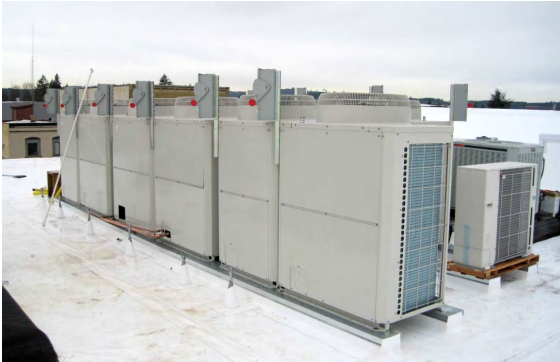
Figure 4-19 VRF Systems Installed at Site C
