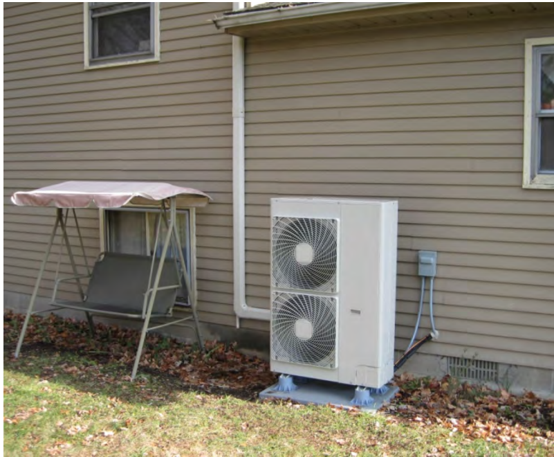
Figure 5-7 Outdoor Unit at the Utility B Site (Refrigerant Lines Hidden by the Gutter Line-Hide)
