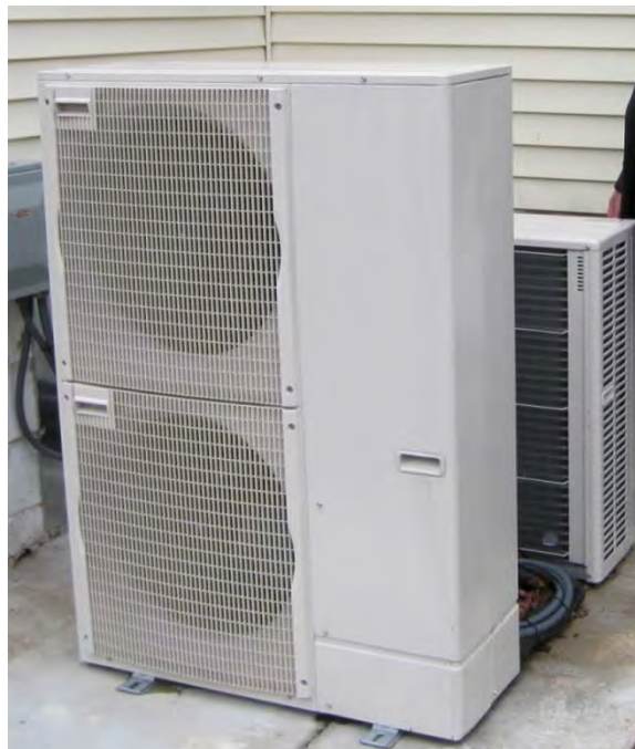
Figure 5-3 Two Variable-Capacity Heat Pumps at a Utility A Site
