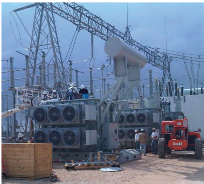
Figure 1. Installation of the three single-phase prototype high-voltage Recovery Transformers at CenterPoint Energy in March 2012.
