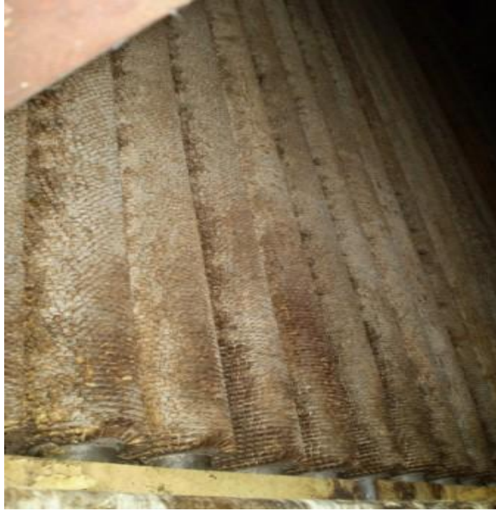
Figure 3-1 Economizer Tube Corrosion Example
