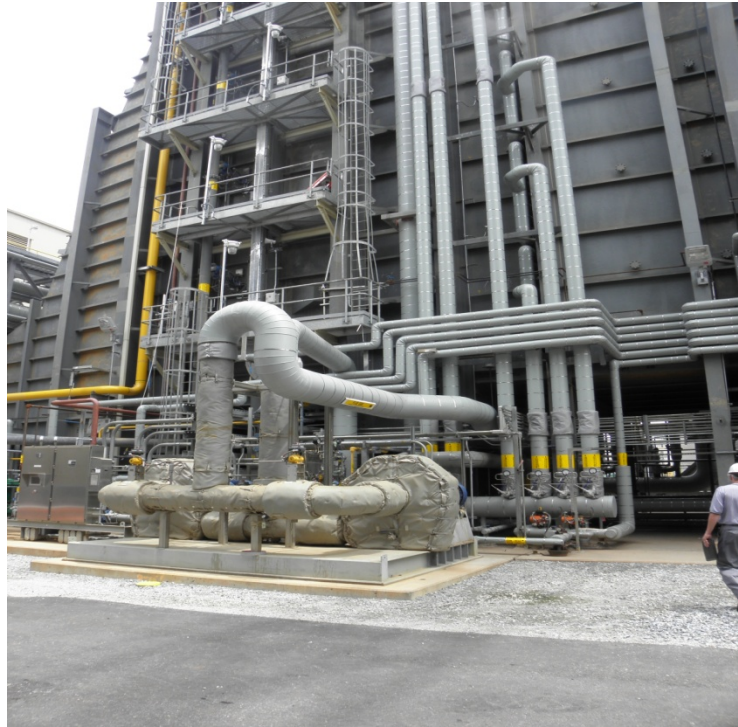
Figure 4-2 Ammonia Mixing Skid Example
