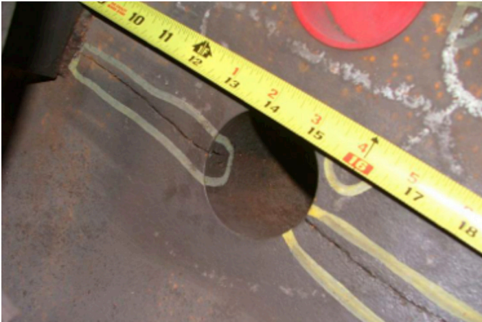
Figure 6 – Cold feedwater introduced to a hot header caused thermal fatigue cracking in this economizer header (courtesy of EPRI).
