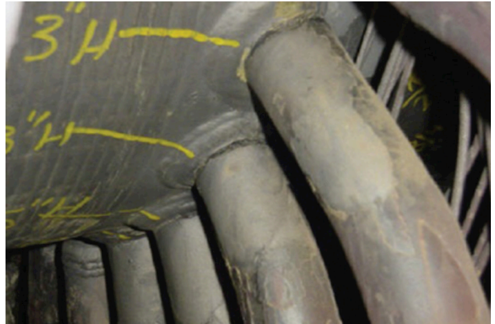
Figure 7 – Waterwall damage caused by corrosion fatigue is often found in steam generators (courtesy of EPRI).
