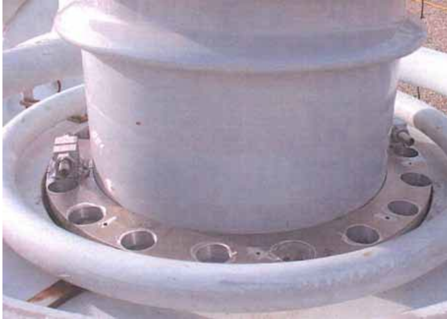
Figure 5–2 Aluminum hub clamp installed over an SF 6 gas leak on a 345-kVb breaker bushing.
