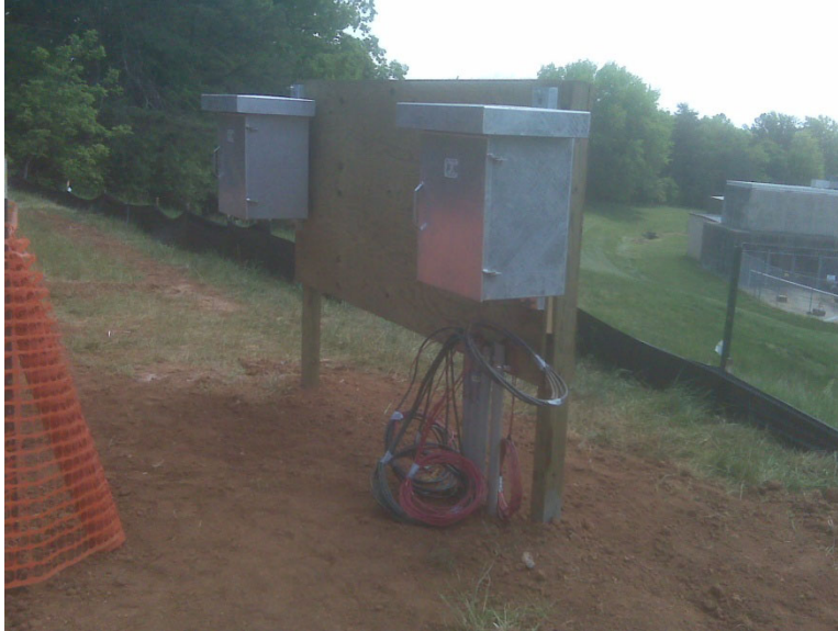
Figure 5-6 Dual rectifiers installed at the Charlotte Underground Transmission Test Facility
