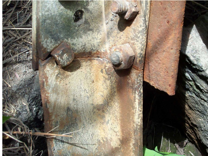
Figure 2-7 Illustration of fatigue damage on a transmission tower leg
