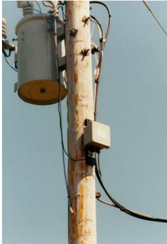
Figure 5-4 Galvanic decoupler (Dairyland) for dc corrosion mitigation
