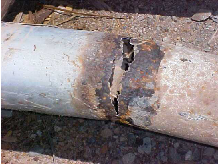
Figure 2-9 Internal corrosion damage on a pipe
