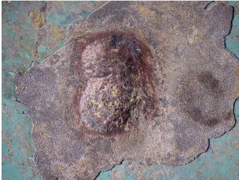
Figure 2-15 Illustration of ac corrosion damage on a pipeline
