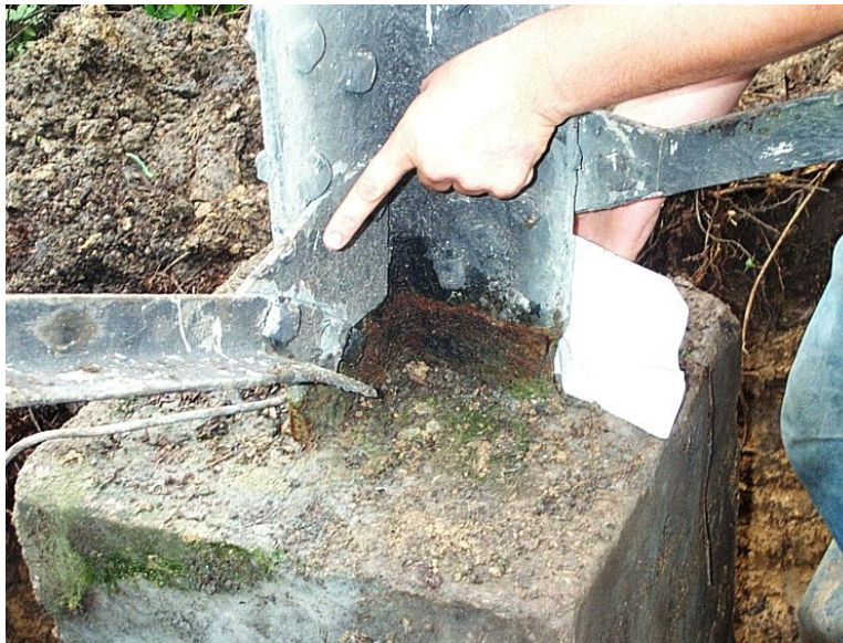
Figure 2-3 Concentration cell corrosion on a stub angle configuration
