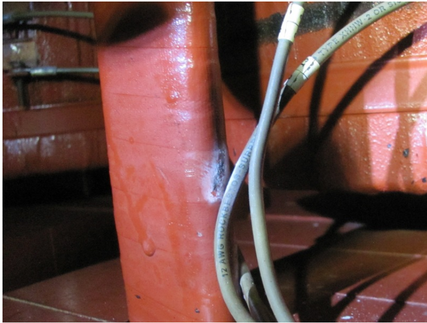
Figure 1-12 Partial arc indication on current transformer cable and phase bar of a 13.8-kV motor
