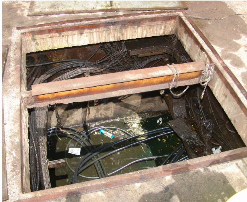
Figure 1-1 Below-grade vault in yard partially filled with water
