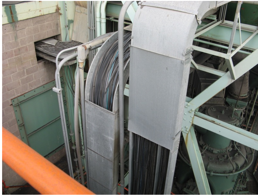
Figure 1-13 Missing cable tray covers expose cables to UV radiation in sunlight
