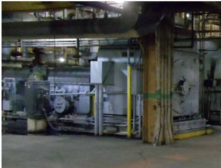
Figure 1-8 Power cable properly routed away from heat vents on 48-year-old motor
