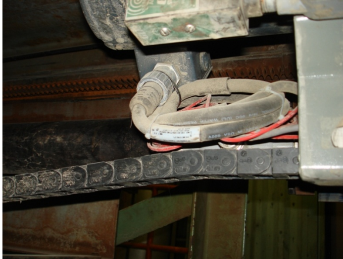
Figure 1-3 Power cable tightly rolled due to excess length in prefabrication
