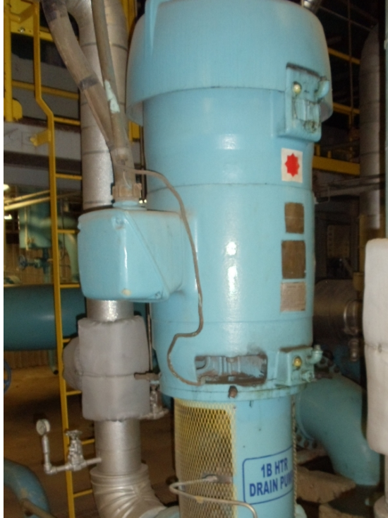
Figure 1-9 Junction box leads poorly placed immediately below the discharge vent hood
