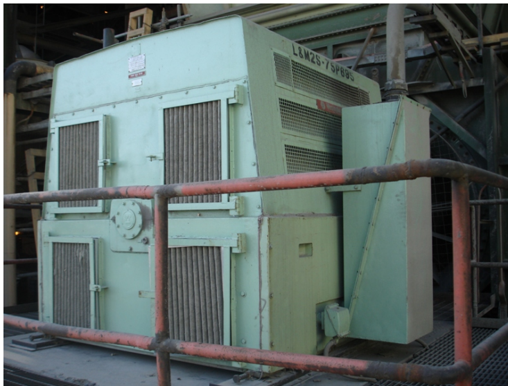
Figure 1-10 Junction box and leads poorly designed in exhaust flow
