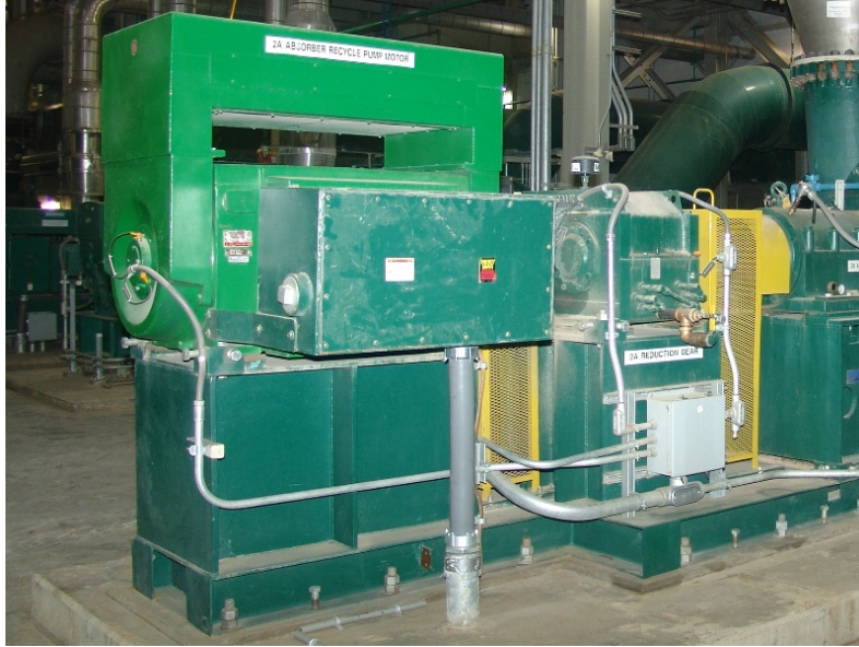
Figure 1-7 Properly routed power cable not in heat exhaust
