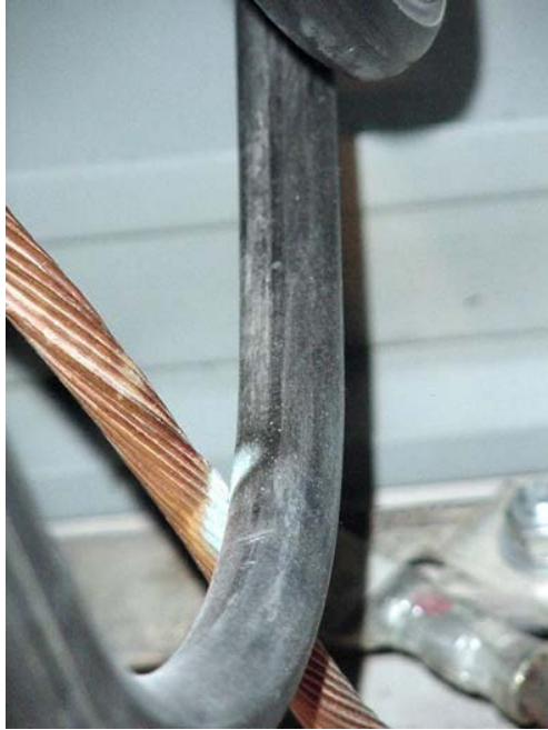
Figure 1-11 Corona discharge indication on a cable and ground
