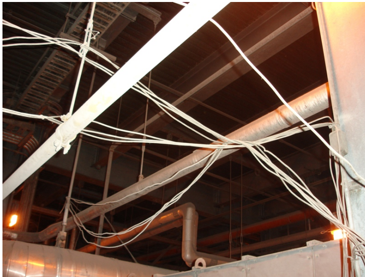
Figure 1-4 Poorly run DCS cable back-fit modification
