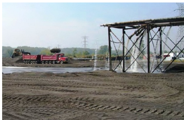
Figure 1-3 Bottom ash sluice lines [11]
