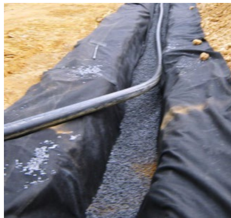
Figure 1-8 Groundwater underdrain (courtesy FirstEnergy)
