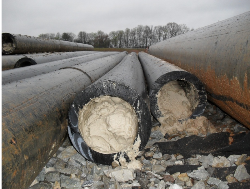
Figure 8-12 Clogged FGD leachate collection piping [Courtesy of TVA]
