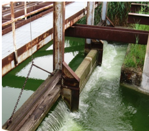
Figure 1-10 Stop logs (courtesy DTE Energy)
