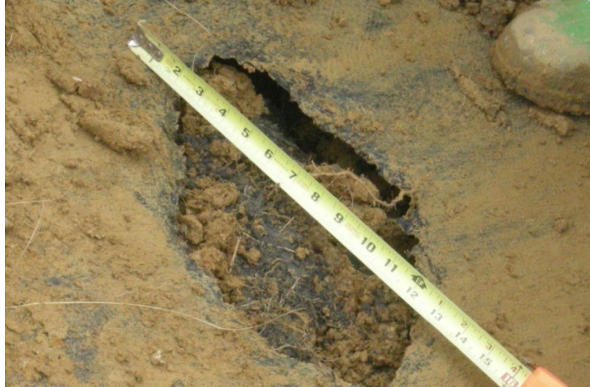
Figure 10-1 Example of a torn geomembrane cap caused by differential settlement
