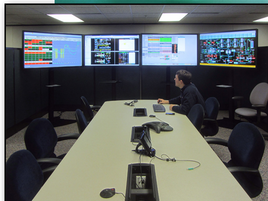
Duke Energy's Central M&D Center in Charlotte, NC uses SmartM&D technology to remotely monitor and assess plant equipment condition.
