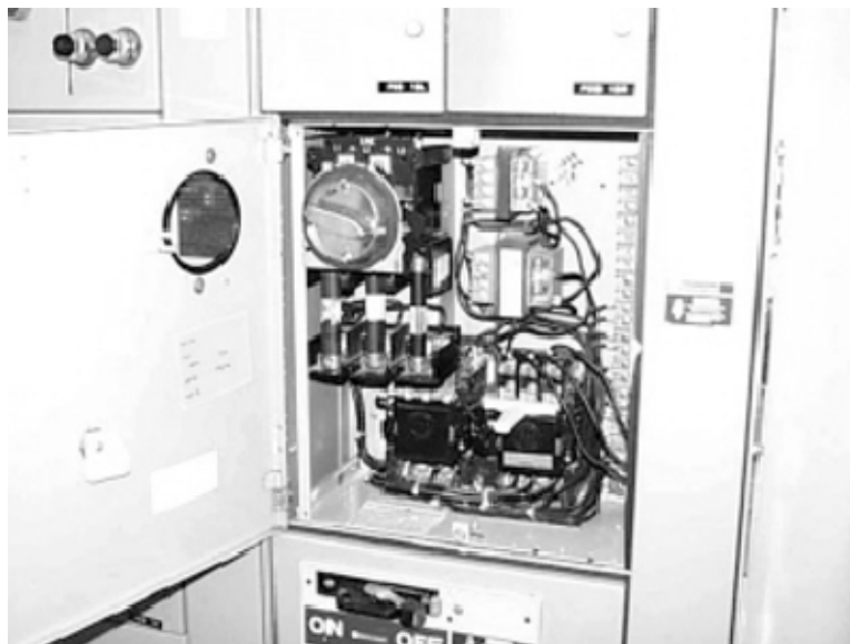
Figure 5-3 Electrical breaker enclosure
