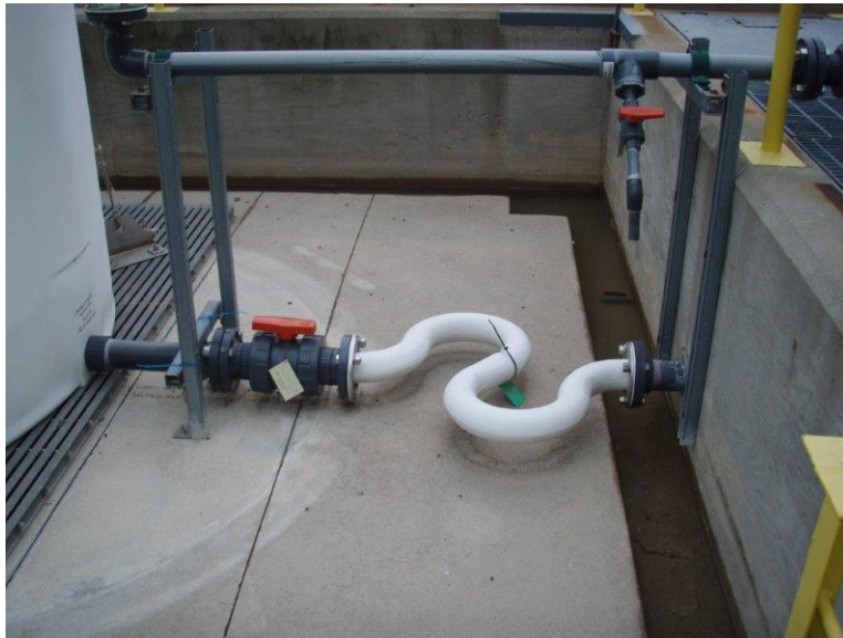
Figure 5-2 A tank discharge connection, stress relief Used with permission from Exelon, Ginna
