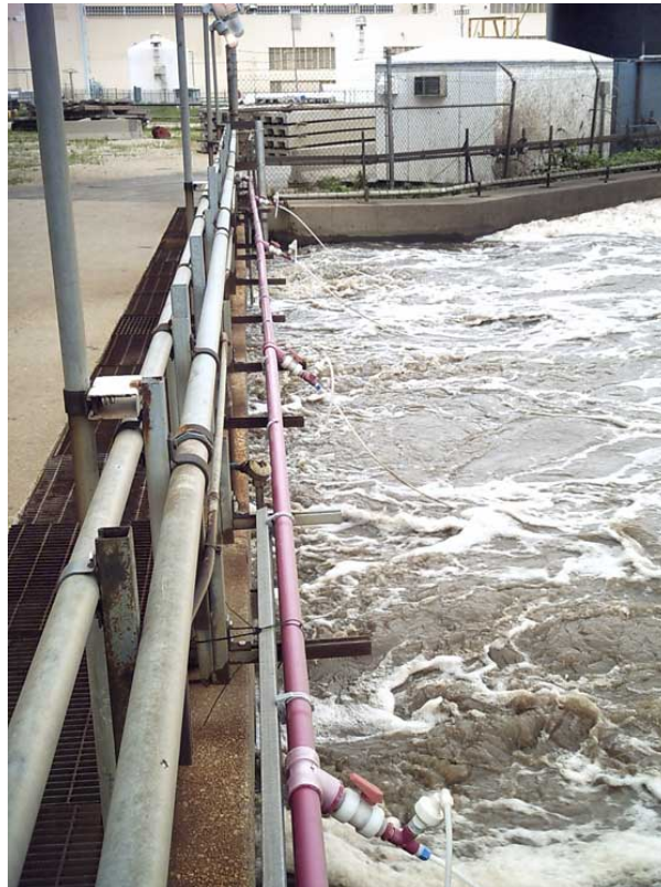
Figure 6-6 A gravity acid feed system Used with permission from Exelon Corporation
