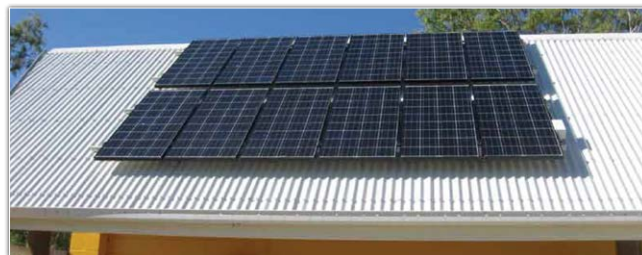
Figure 1 – Example of rooftop solar installation
