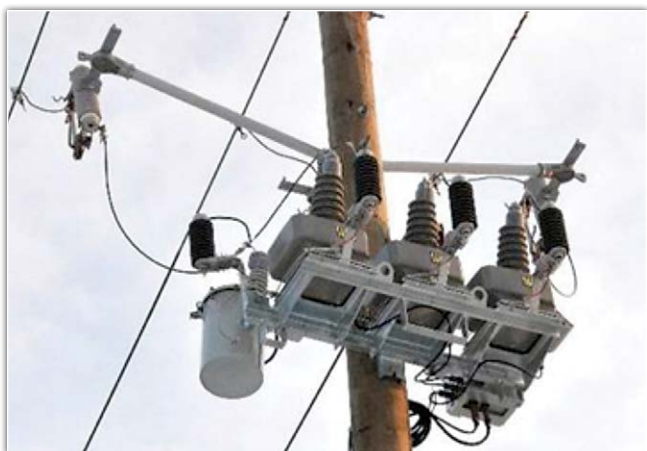
Figure 1 – Medium voltage monitoring stations
