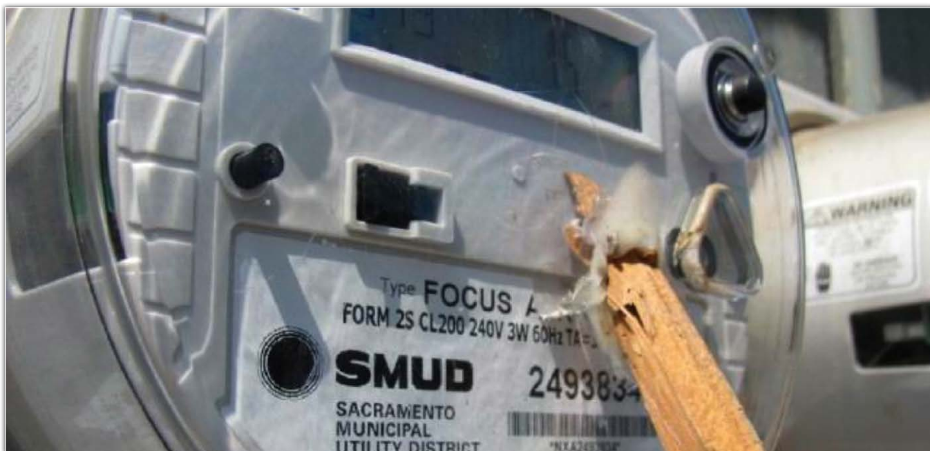
This is an example of attempted power theft. The customer drilled through the meter cover to install a stick on a button that is used to place the meter in a diagnostic mode.
