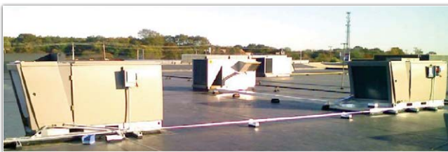
Figure 1 – Ice Bear installation on roof of big box retailer
