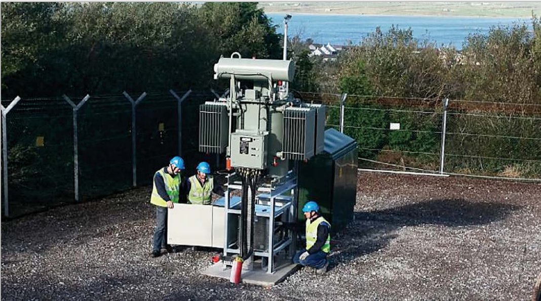
Arc suppression system at Gurrane Substation
