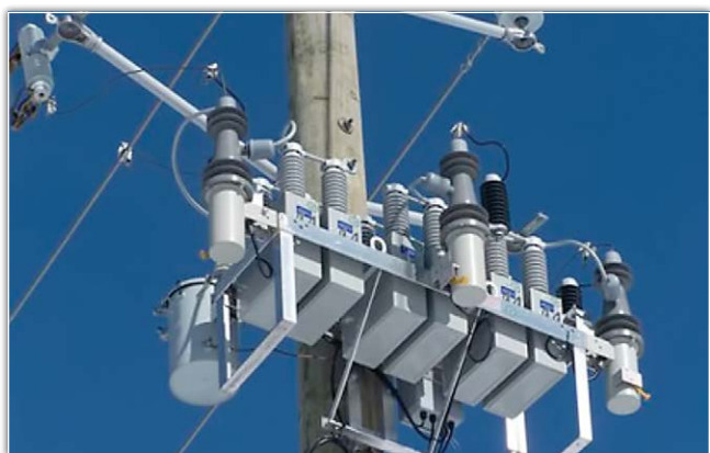
Figure 2 – Automated distribution capacitor banks
