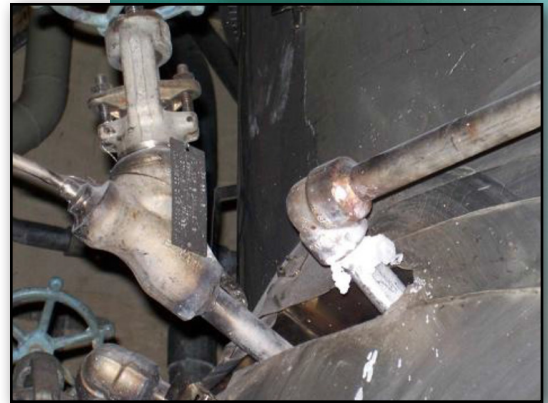
Weld overlay was applied to a socket weld in the reactor coolant system at AEP's DC Cook nuclear plant.
