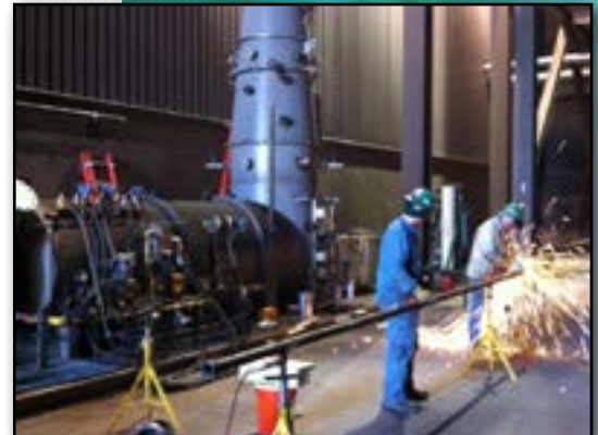
Sparks fly as the Great River Energy team starts SAP installation at Coal Creek Station.
