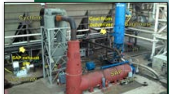
The AEP/SWEPCO H.W. Pirkey Power Plant SAP system.
