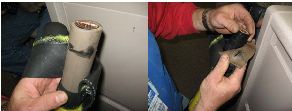
Figure 7-6 New splice of a 15-kV cable operated at 13.8-kV that failed at the 12-kV \tan \delta step prior to the 16-kV withstand test
