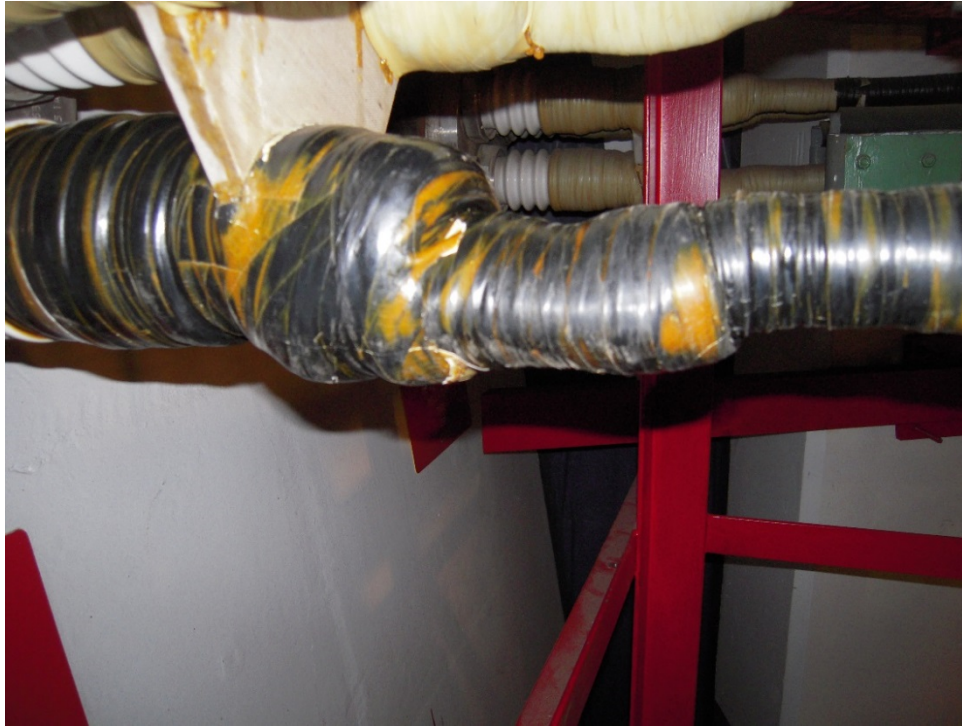
Figure 4-4 Noticeable overheating of the C phase penetration. Note the tan color of the parallel cables in the background.
