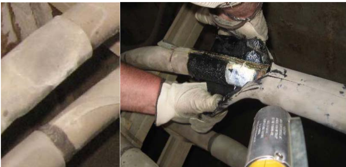
Figure 7-5 Splice with a poor heat shrink being opened and exposing the degraded zinc metallic insulation shield
