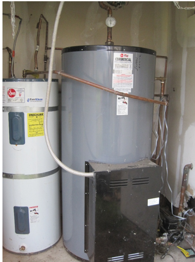
Figure 3-1 Existing Water Heating Setup
