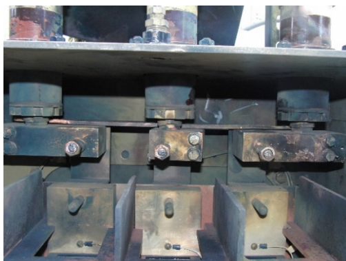
Test ID 62: 3Φ bar back fuse terminal
