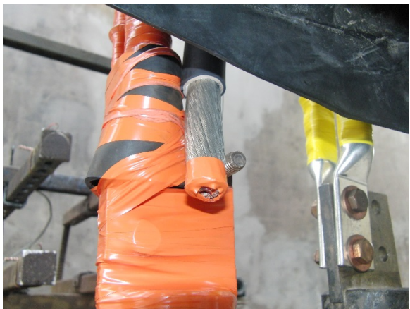
Test ID 55: CΦ-BΦ cable; 1.57 cycles
