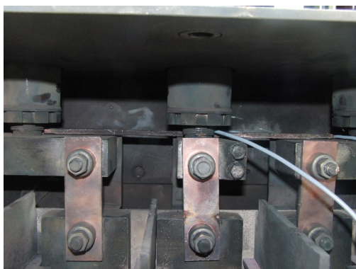
Test ID 64: 3Φ bar back fuse terminal
