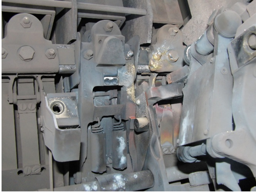
Figure 2-10 Post Test ID 65: Damage at the circuit breaker
