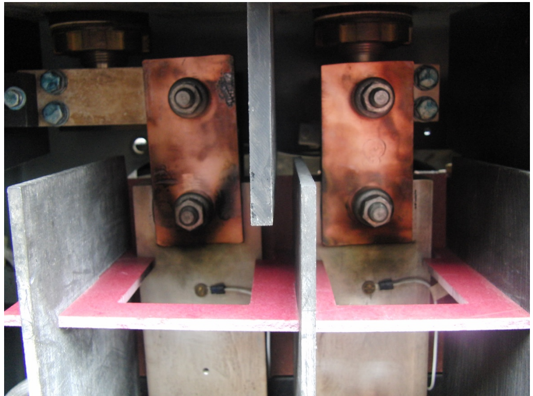
Figure 4-11 Arcing inside NP2 at fuse terminal location C \Phi left-B \Phi right
