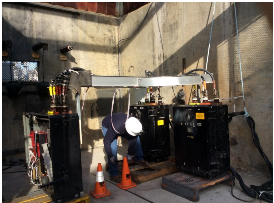
Figure 1-5 Side view of network protector setup
