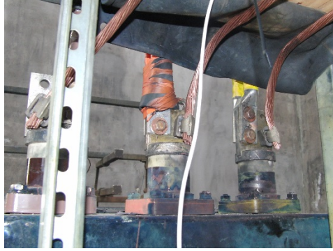
Cables attached to NP3
