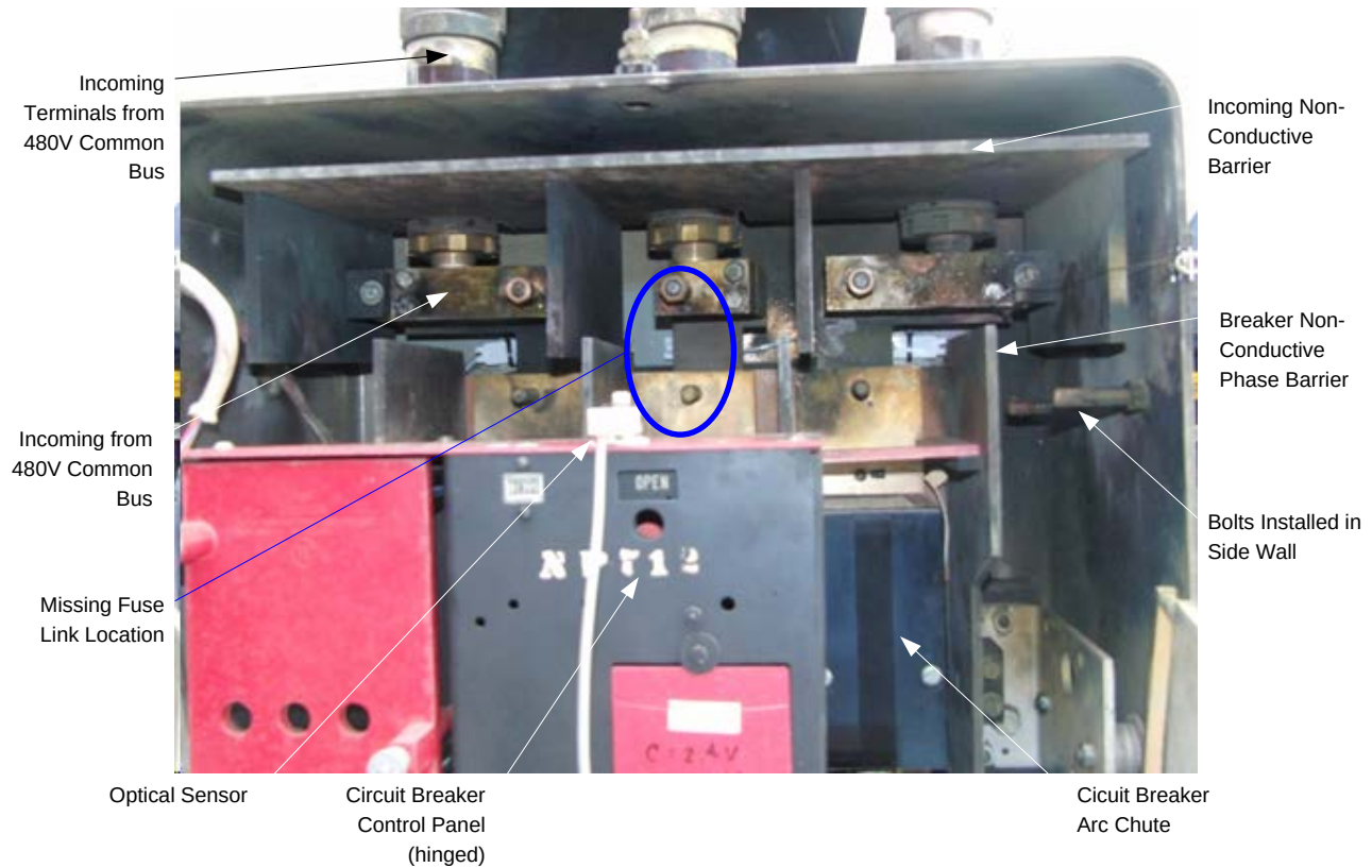
Figure 2-1 Interior NP3 with the non-conductive barrier installed
