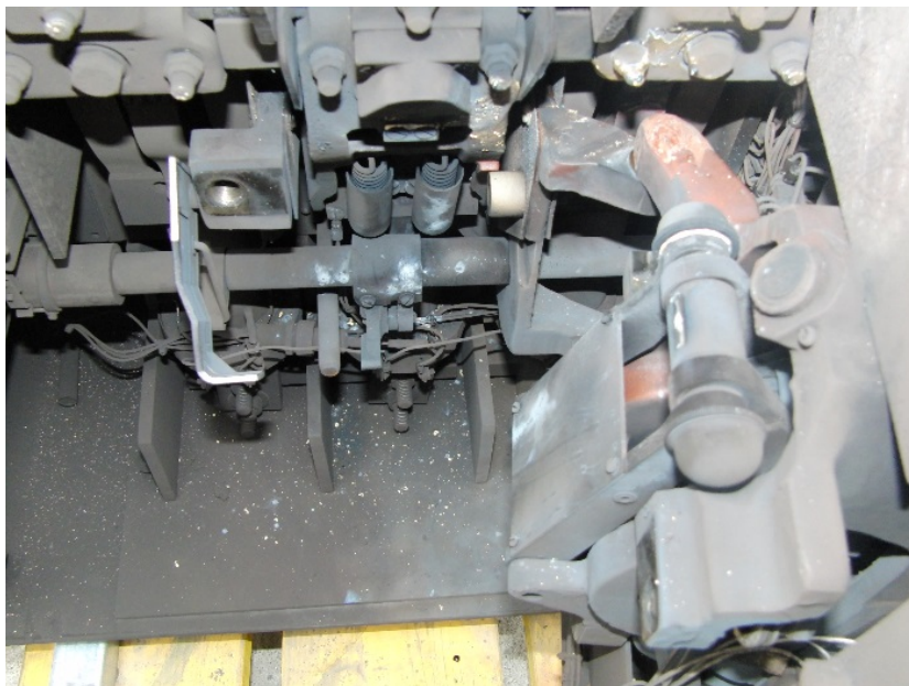
Figure 2-11 Post Test ID 65: Damage below arc chutes, behind the control module
