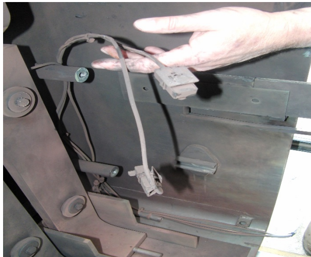
Figure 4-10 Post Test 65: Condition of the omnidirectional sensors on the back wall
