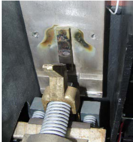
Pre-Test ID 60: Arcing Contact
