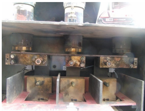
Test ID 61: 3Φ bar front fuse terminal
