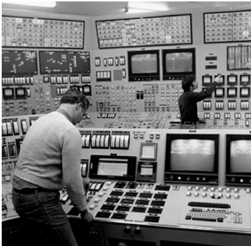
Figure 2-1 Old KCP&L Control Room
