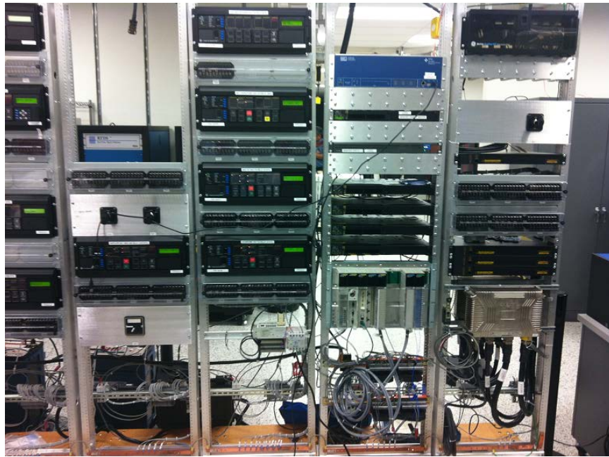
Figure 3-3 SCE Substation Automation Lab
