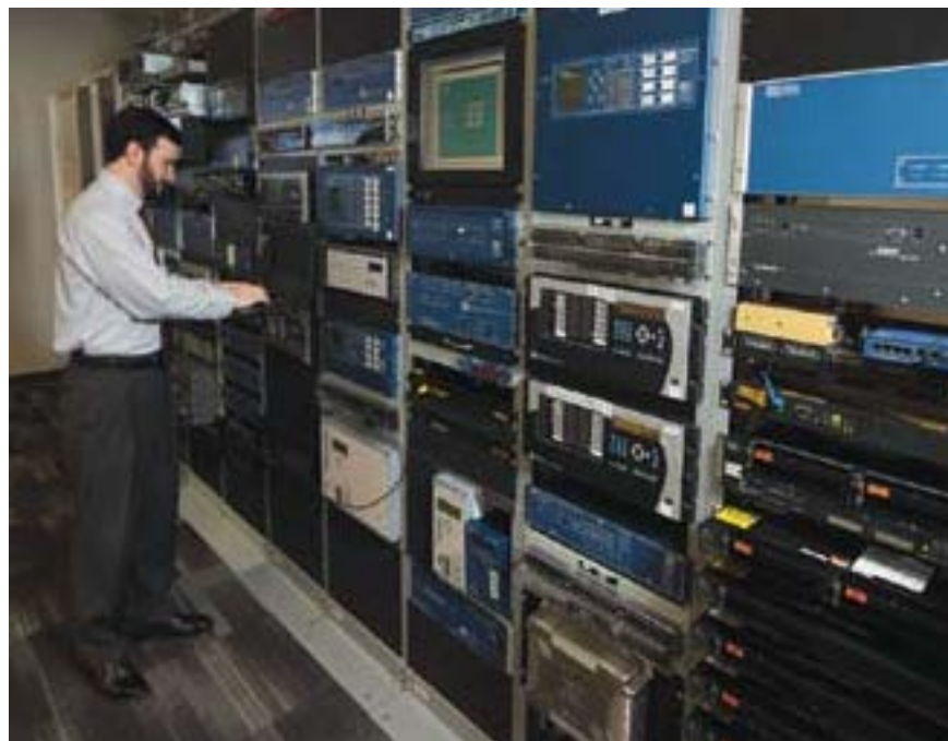
Figure 3-1 Burns & McDonnell Smart Grid Lab
