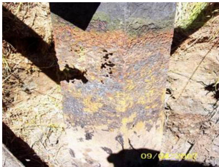
Figure 2. Below grade corrosion of steel tower Source: Public Utilities Maintenance
