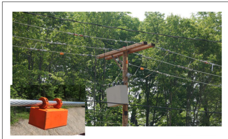
Figure 12-1 Prototype conductor sensor on distribution automation installation
