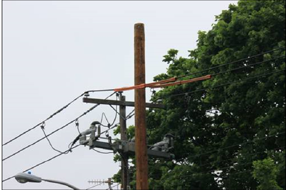
Figure 5-2 New class H1 pole being installed on an existing DA switch location
