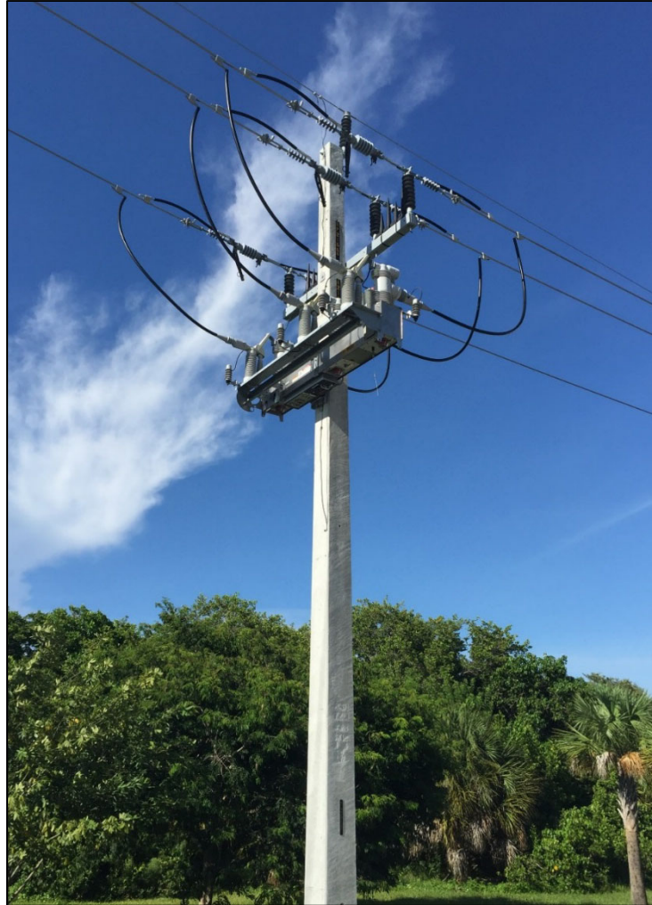
Figure 5-3 DA switch on concrete pole
