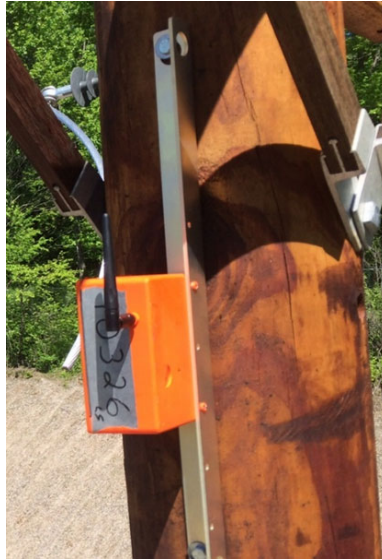
Figure 12-6 Example of a prototype sensor installed on a pole
