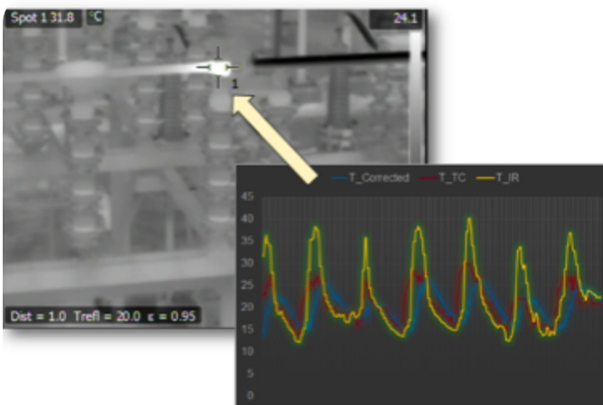
Figure 8 – IR Measurements from an Online Substation Monitoring System, Corrected Using EPRI-Developed Algorithms
