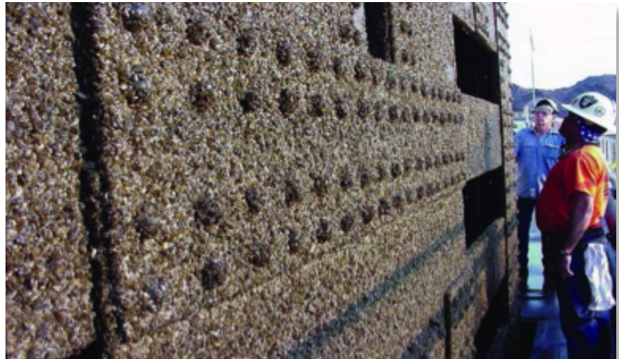
Intake gate structure fouled with invasive mussels (image courtesy of U.S. Bureau of Reclamation).
