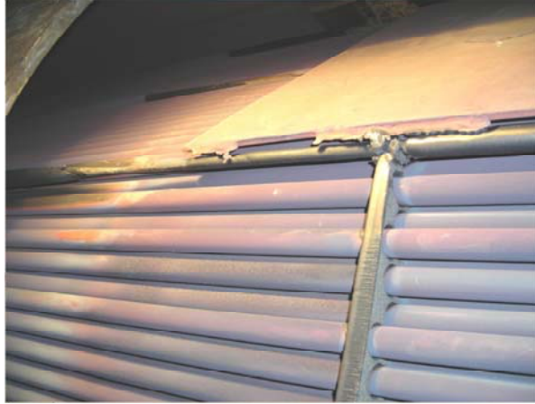
Figure 2-2 Feedwater Heater Impingement Plate
