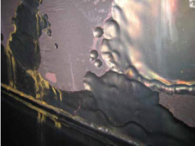
Figure 6-2 Feedwater Heater Shell – Steam Cutting Erosion [16]
