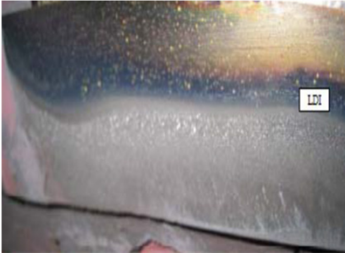
Figure 4-3 Heater Shell Surface Damage from Liquid Droplet Impingement [15]
