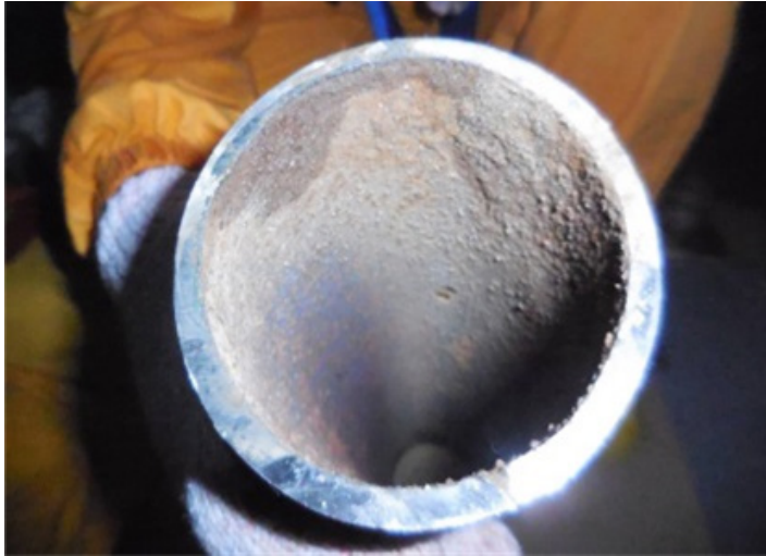
Figure 2-27 Core Spray System Component – Cavitation Erosion (Photo Courtesy of Taiwan Power)
