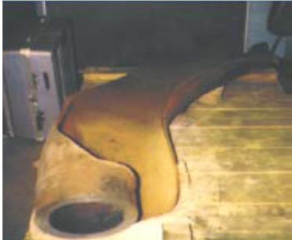
Figure 9-6 Ruptured Feedwater line to Economizer at Fossil Power Plant [28]
