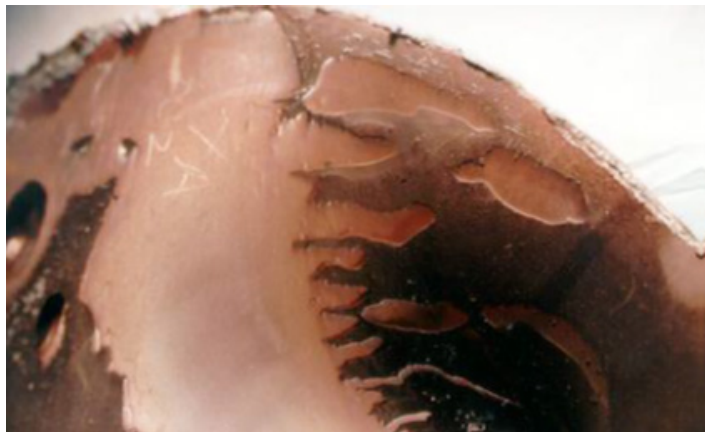
Figure 8-1 Pipe Damage – Two Phase Flow Accelerated Corrosion [11]
