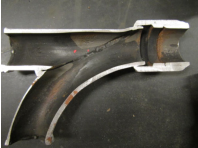
Figure 7-9 Socket Welded Fitting in Drain Line – Single Phase Flow Accelerated Corrosion [23]
