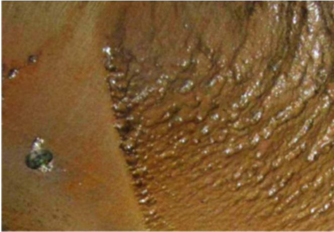
Figure 2-12 High Pressure Core Spray – Close-Up of Degraded Surface - Cavitation and Flow Curvature Erosion [3, 20]
