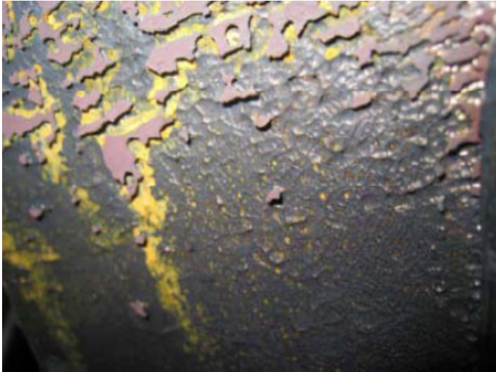
Figure 8-5 Feedwater Heater Shell – Two Phase Flow Accelerated Corrosion [15]
