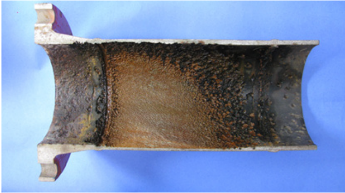
Figure 2-4 Fire Protection Downstream of Orifice - Cavitation Erosion [14]
