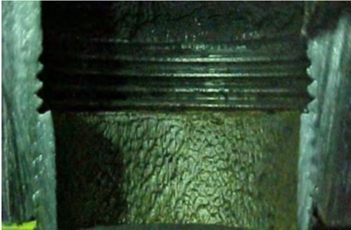
Figure 10-2 Low Temperature FAC – Reactor Building Closed Loop Cooling Showing Scalloped Surface [6, 25, 27]
