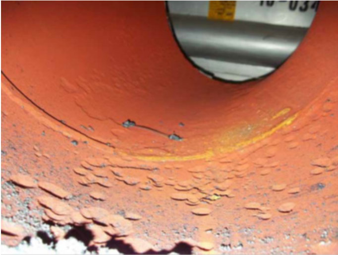
Figure 2-10 Heater Drains - Cavitation Erosion [20]
