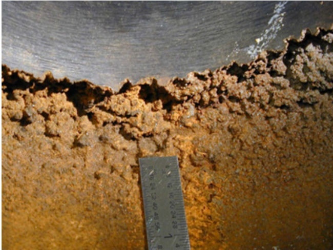
Figure 2-8 Close-Up View of Degraded Surface of WP22 Fitting - Cavitation Erosion [3, 18]
