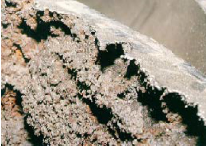
Figure 4-2 Magnified View of Surface Degradation from Liquid Droplet Impingement [11]
