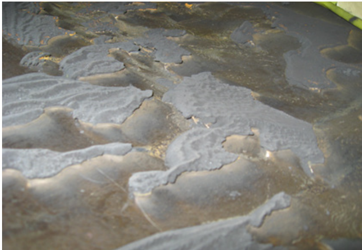
Figure 8-4 Feedwater Heater Shell Wear – Two Phase Flow Accelerated Corrosion [14]
