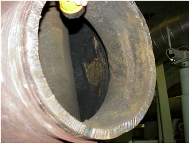
Figure 2-24 Feedwater Regulating Valve Body – Cavitation Erosion [3]
