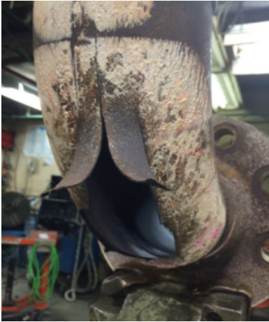
Figure 8-12 Reheat Steam and Moisture Separator System Elbow Downstream of Orifice – Two Phase Flow Accelerated Corrosion [24]
