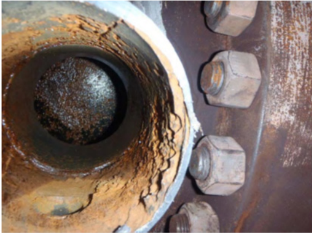
Figure 7-10 Reactor Water Clean Up Heat Exchanger Nozzle and Pipe – Single Phase Flow Accelerated Corrosion [25]
