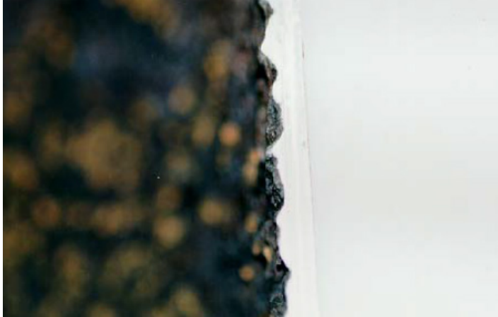
Figure 2-3 Profile of Pipe Surface Damage from Cavitation Erosion [11]
