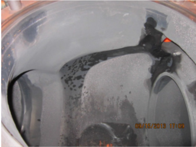
Figure 8-9 Extraction Steam Wear in Non-Return Valve Body – Two Phase Flow Accelerated Corrosion [21]
