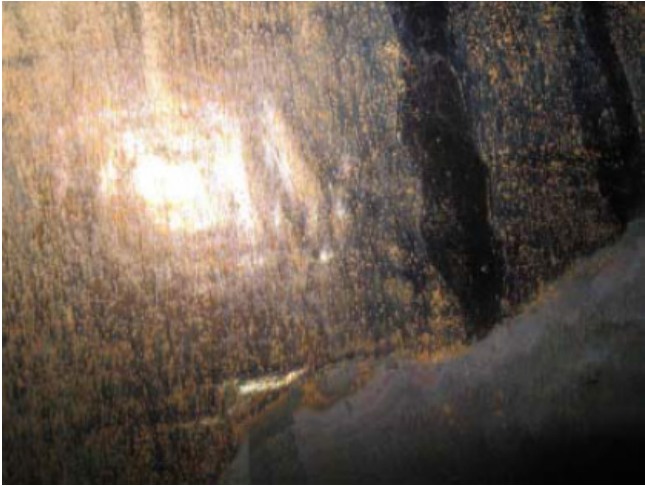
Figure 5-2 Feedwater Heater Shell – Solid Particle Erosion [15]
