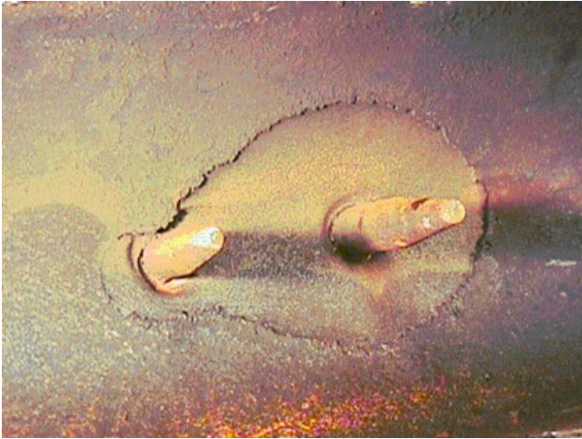
Figure 7-14 Damaged Pipe Wall at Thermowells – Single Phase Flow Accelerated Corrosion [7]
