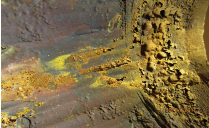
Figure 2-31 Condensate Cooling Water – Cavitation Erosion (Photo Courtesy of PG&E)
