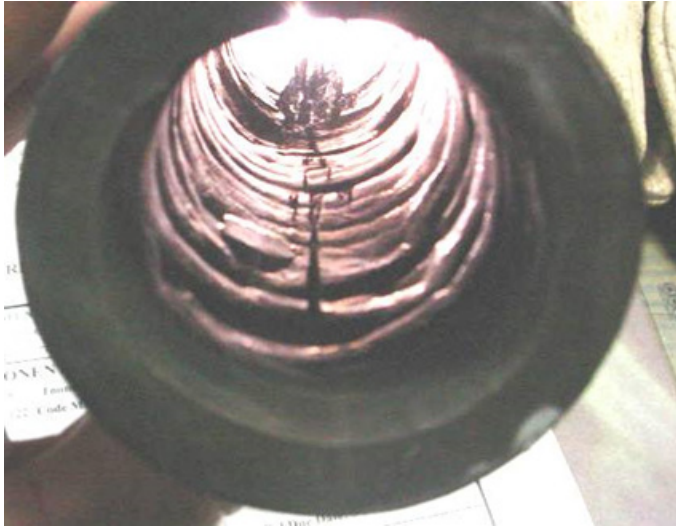
Figure 5-7 Steam Generator Blowdown System – Solid Particle Erosion [3, 8]
