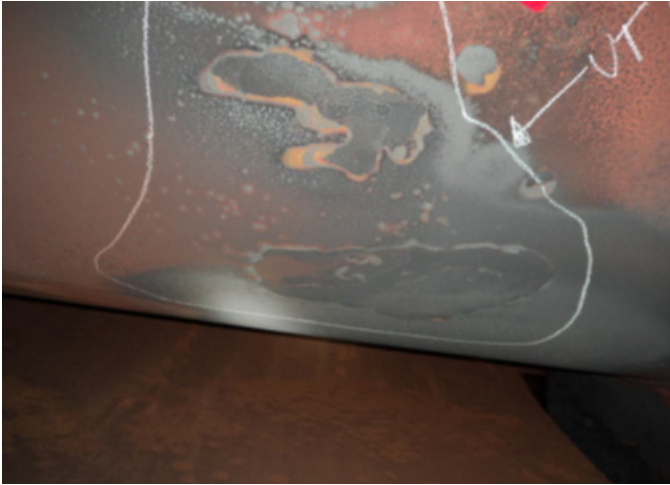
Figure 8-8 Low Pressure Feedwater Heater – Two Phase Flow Accelerated Corrosion [18]
