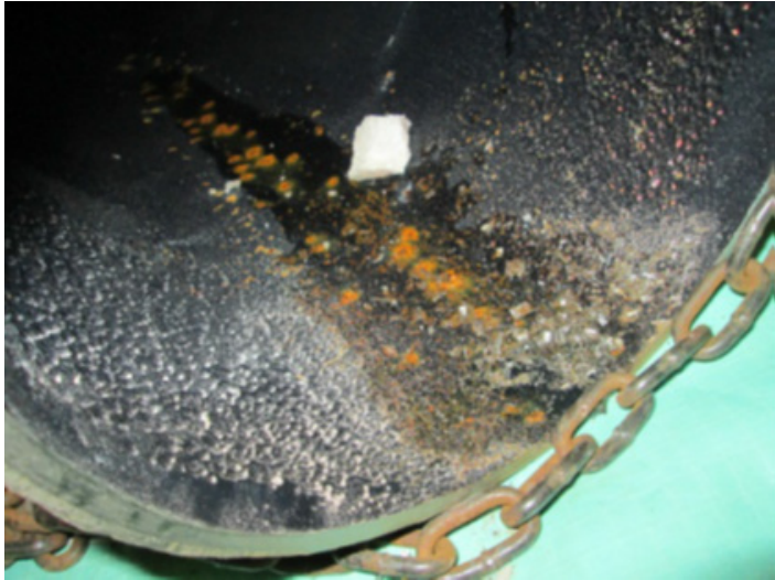
Figure 2-15 Heater Drains Downstream of Check Valve – Cavitation Erosion and Flow Accelerated Corrosion [22]
