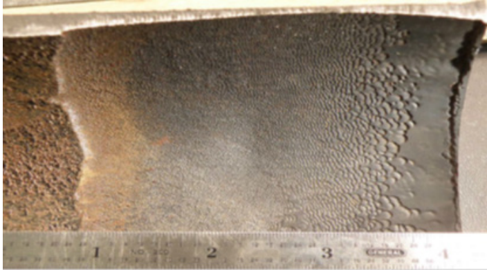
Figure 8-7 Steam Supply to Gland Steam – Two Phase Flow Accelerated Corrosion and Liquid Droplet Impingement Erosion [17]
