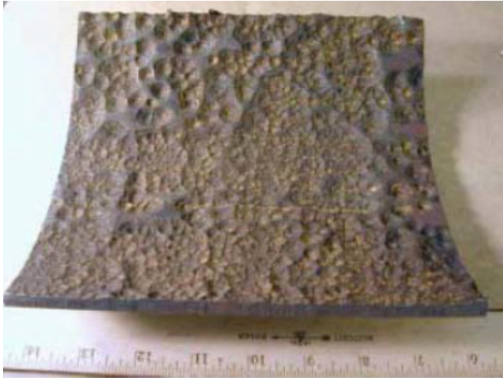
Figure 10-9 Degradation of Pipe Surface in the Condensate System Downstream of the Polishers [6]
