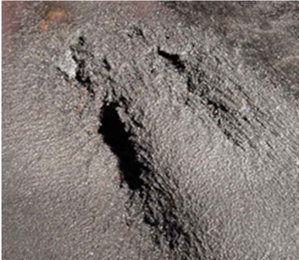
Figure 4-13 Piping Downstream of a Normally Closed Bleed Line Valve which was Leaking By [3, 8]
