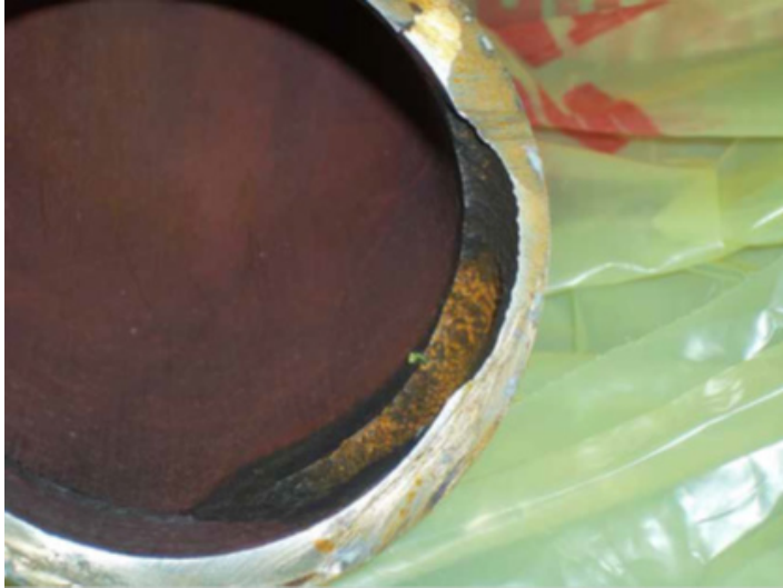
Figure 7-5 Reactor Water Clean Up – Close Up View of Wall Loss - Single Phase Flow Accelerated Corrosion [20]
