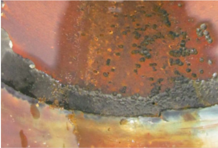
Figure 10-1 Low Temperature FAC – Polisher Piping between Isolation Valve and Resin Trap [24]
