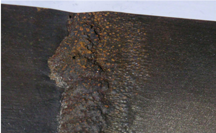
Figure 2-19 Feedwater Recirculation Line to Condenser – Cavitation Erosion [3, 8]
