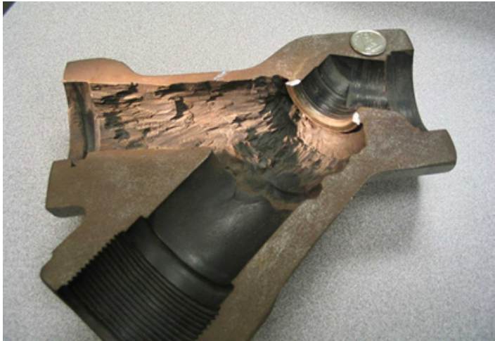
Figure 5-4 Boiler Blowdown Valve Body – Solid Particle Erosion [3, 20]
