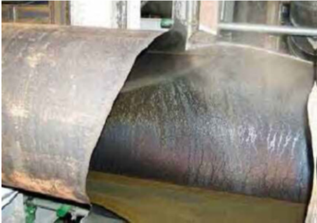
Figure 7-6 Condensate Line Downstream of Flow Measuring Orifice – Mihama Unit 3 Single-Phase Flow Accelerated Corrosion [20]
