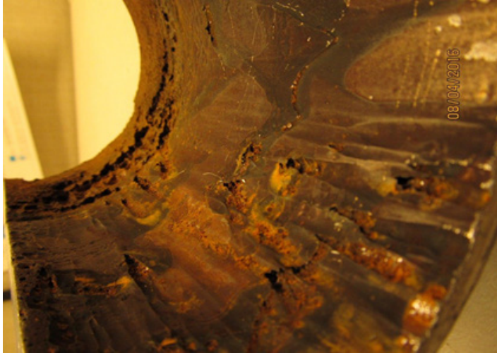
Figure 2-29 Condensate Cooling Water – Cavitation Erosion (Photo Courtesy of PG&E)
