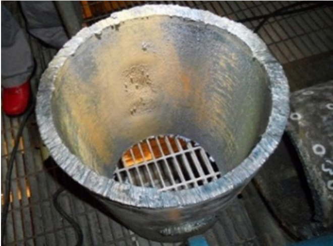
Figure 3-4 Heater Drain System – Flashing Flow Erosion (Photo Courtesy of Taiwan Power)
