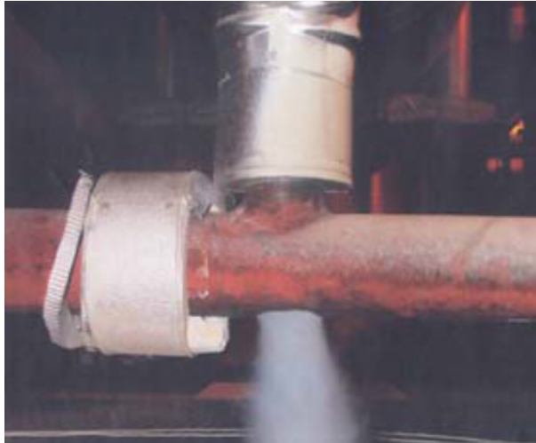
Figure 4-11 Turbine Stop Valves and 'B' Moisture Separator Re-heater (MSR) cross-under piping drains to the Condenser [23]
