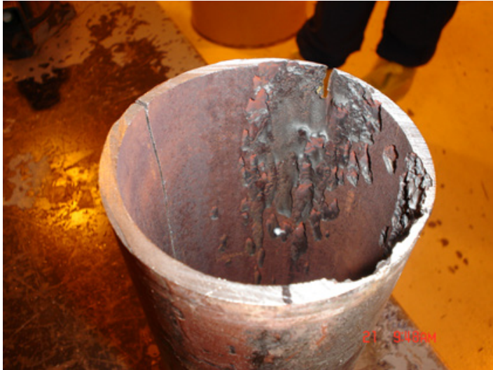
Figure 2-5 Pipe Downstream of Control Valve - Cavitation Erosion [14]
