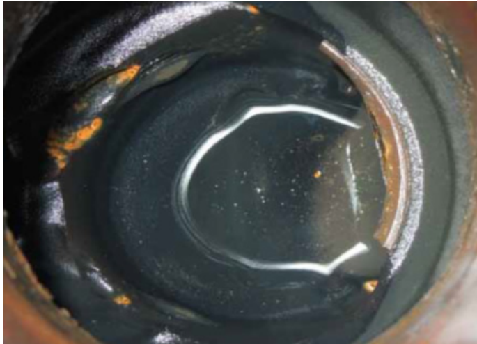
Figure 4-8 Reactor Water Clean-Up (RWCU) Valve Body Leak and Internals LDI [20]
