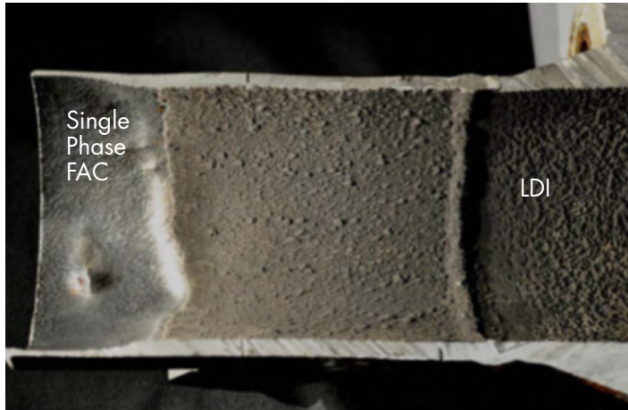
Figure 7-12 Pipe with Two Damage Mechanisms – Liquid Droplet Impingement Erosion and Single Phase Flow Accelerated Corrosion [25]
