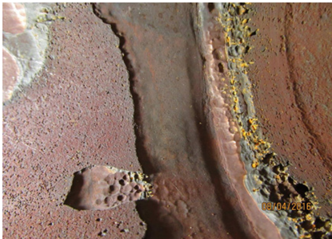
Figure 2-30 Condensate Cooling Water – Cavitation Erosion (Photo Courtesy of PG&E)
