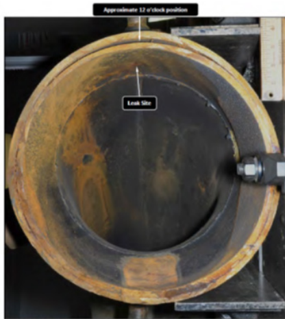
Figure 2: MMS 2HA-8 spool piece, as received (looking in direction opposite to steam flow).
