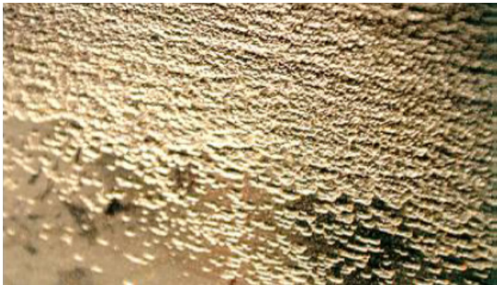
Figure 7-1 Surface Damage – Single Phase Flow Accelerated Corrosion [11]
