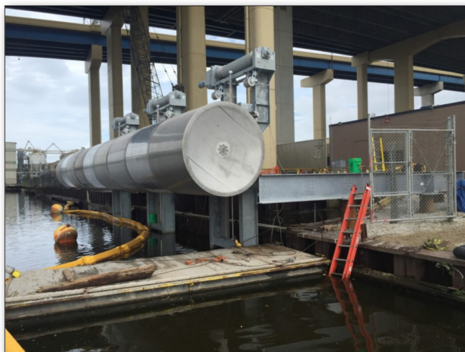
Figure 1. Cylindrical Narrow Slot (2.0 mm) Screens (3) Installed at We Energies Valley Power Plant in Milwaukee, WI [photo courtesy of We Energies]
