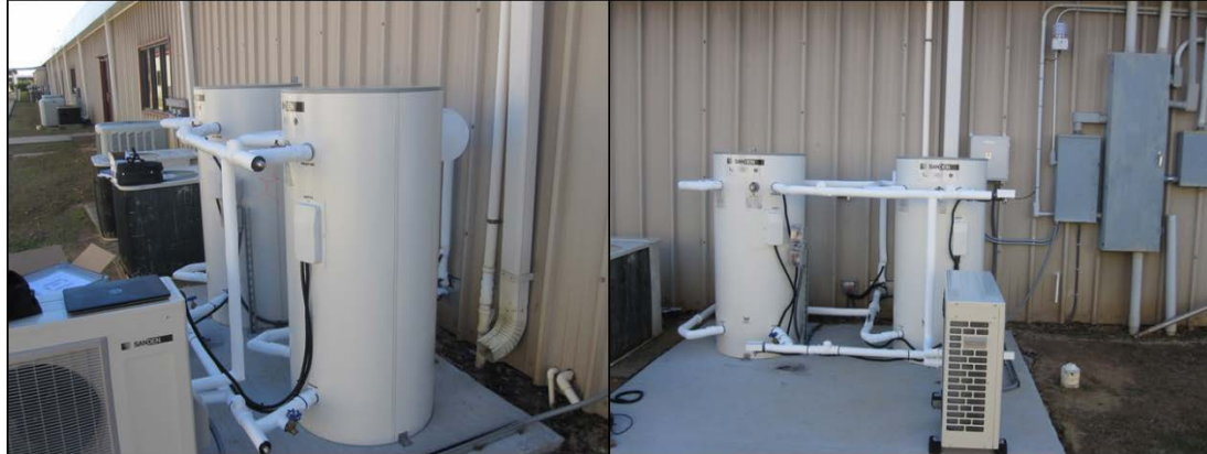
Figure 2-2 HPWH and tanks during installation, showing parallel tank layout
