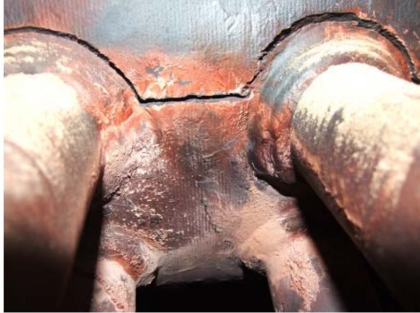
Figure 1-1 Cracked boiler header due to creep/fatigue damage
