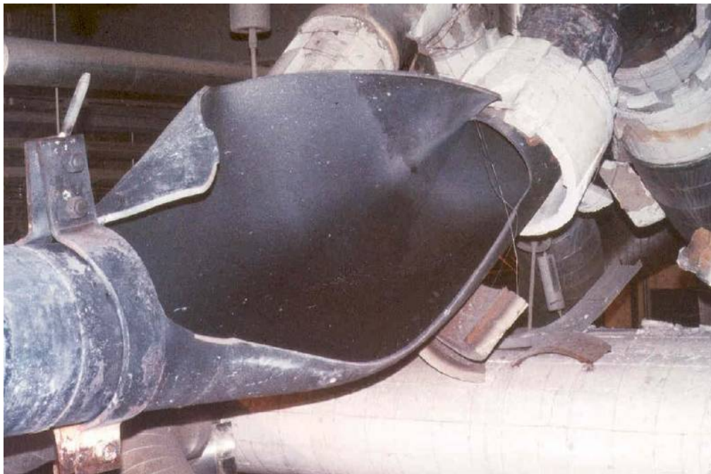
Figure 1-2 Rupture of seam welded high energy pipe
