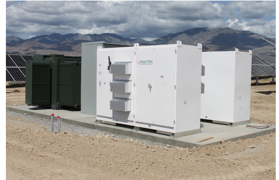
Solectria Inverters for Alamosa Project, Colorado
