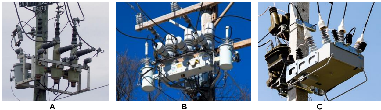
Figure 3-1 Examples of distribution reclosers: G&W Viper-ST (triple-single recloser) [A], Eaton (Cooper) NOVA (three-phase recloser) [B], and Tavrda OSM (three-phase recloser) [C].
