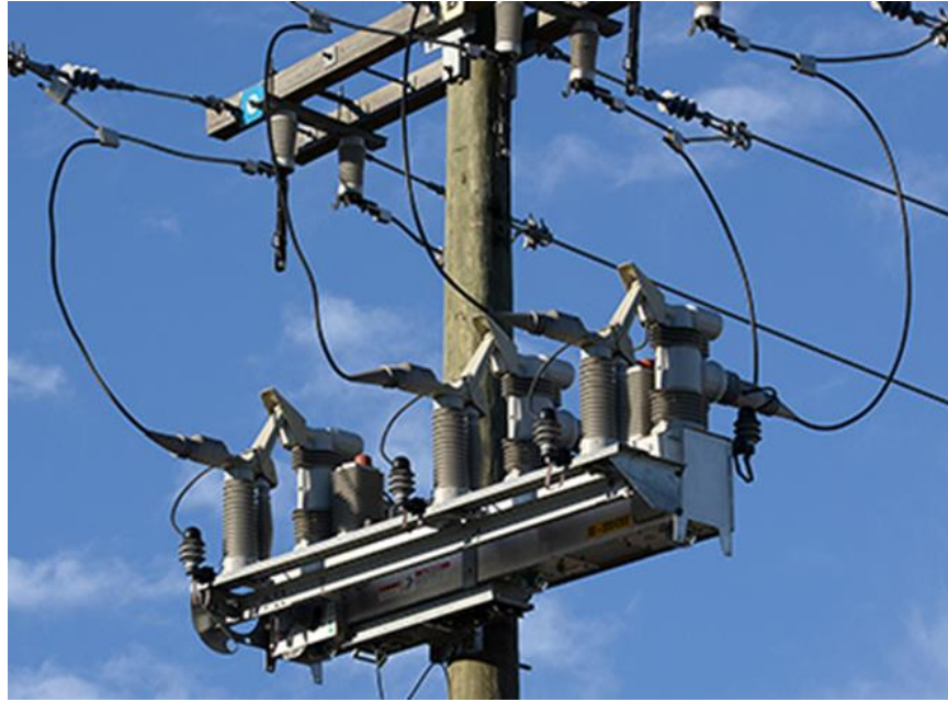
Figure 3-2 Pulse-closing recloser: S&C's IntelliRupter PulseCloser Fault Interrupter
