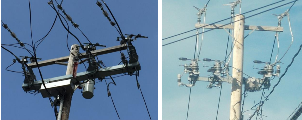
Figure 3-4 Two examples of motor operated air break switches
