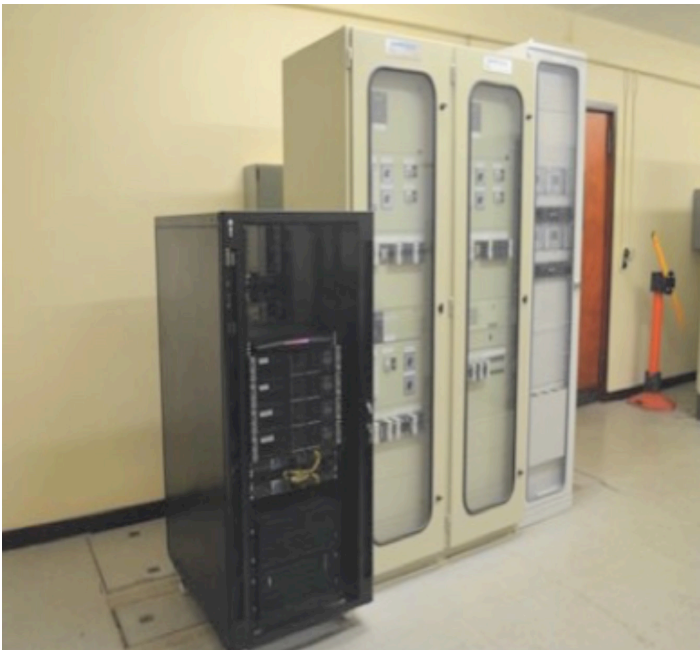
Figure 2 – Controller located at Dunbar GSP (Source: SP Energy Networks)
