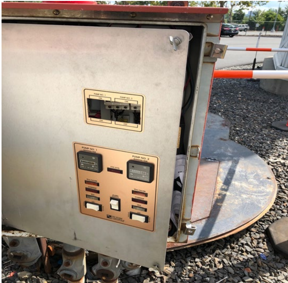
Figure 2-4 Sewage pump controls in manual mode due to loss of level controller
