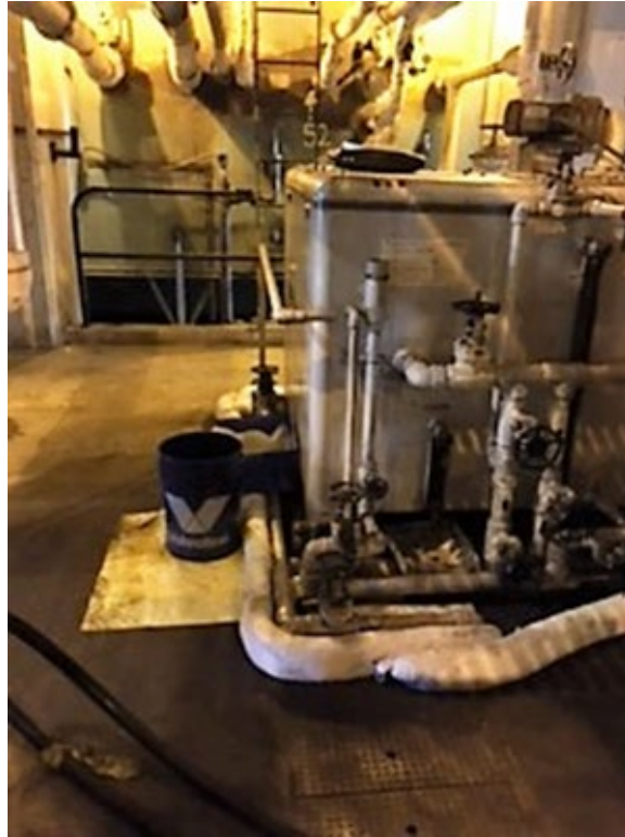
Figure 2-1 Operator manually draining water from lube oil tank once every shift
