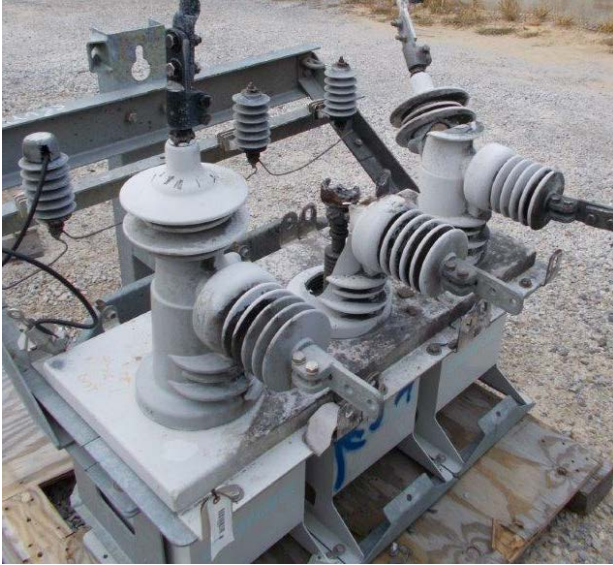
Failed distribution recloser example.
