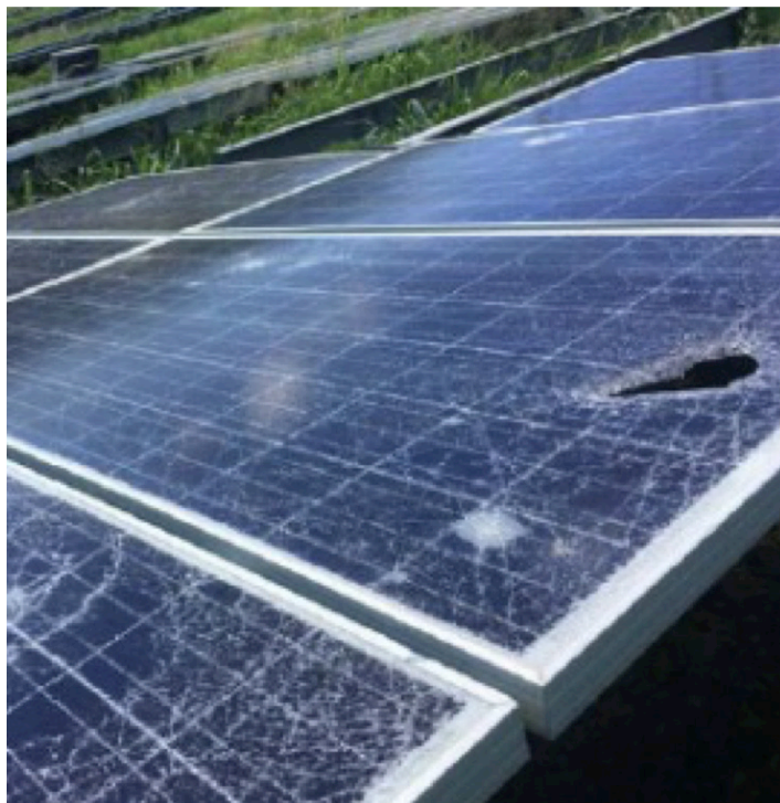
Storm-damaged modules (Photo Credit: Eliza Hotchkiss, NREL)
